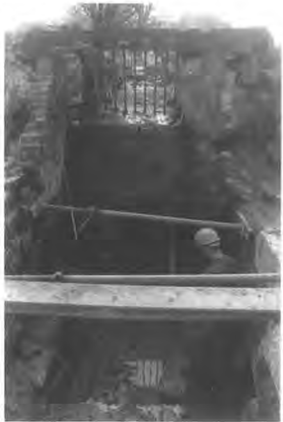
PLATE 3 The drop of the wheel pit, excavated after the mill stream was diverted.
