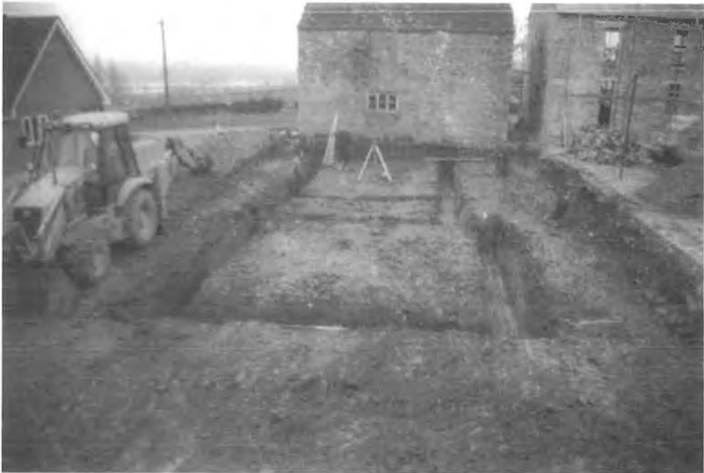
PLATE 2 Excavation area after cutting of wall footings, with granary to rear (looking south).
