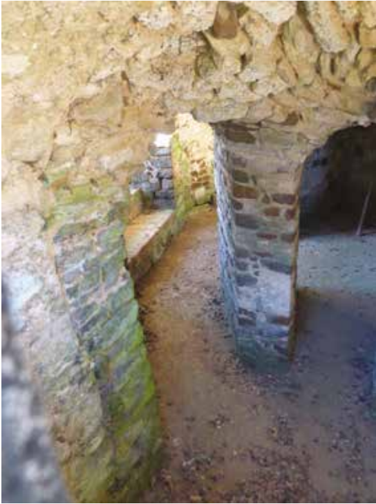
FIGURE 5 View down into crypt through E window. On left, primary jamb of niche with secondary masonry added in front to support vault; centre right, free-standing pier of added vault
