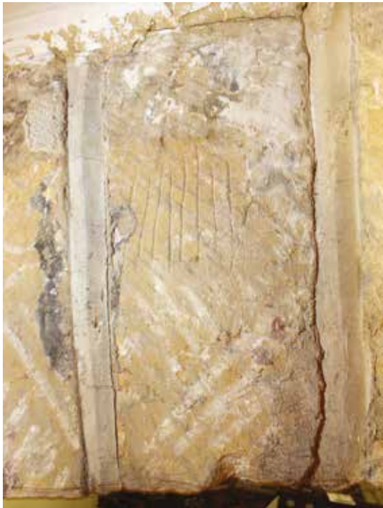
FIGURE 8 Detail of voussoir 10, showing free-hand vertical incisions, perhaps a mason's mark (EH)
