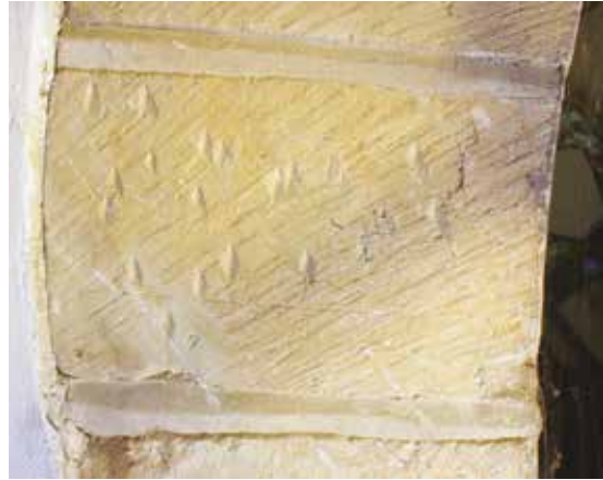
FIGURE 7 Detail of voussoir 5 showing: dressing of the ashlar, incised radial line, and later keying (EH)
