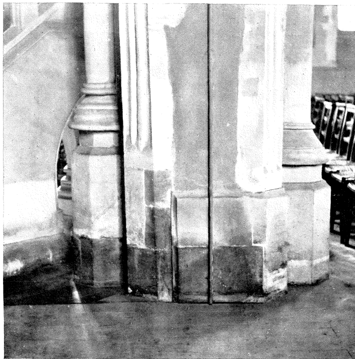
ALL SAINTS CHURCH, HIGH WYCOMBE. BASES OF CHAPMAN'S ARCH (TO LEFT) AND OF THE OLDER ARCADE (TO RIGHT) ON THE NORTH SIDE OF THE NAVE.
