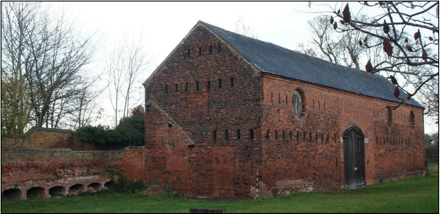
Plate 1: General view of the barn looking north-east. Note the cattle troughs extending along the boundary wall.
