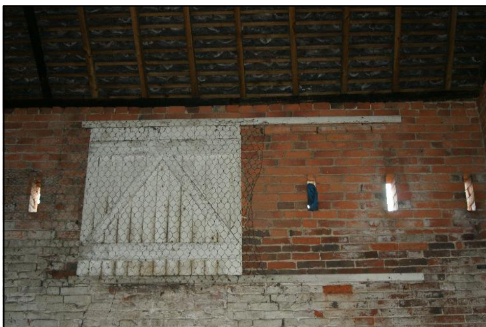
Plate 15: The upper part of the south wall of Bay 3 with the timber shutter and rails of the circular pitching hole, viewed looking south. Note the whitewash Adhering to the brickwork.
