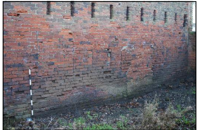
Plate 9: The blocked window, door and ventilation slits in the south elevation of Bay 1, viewed looking south-west.
