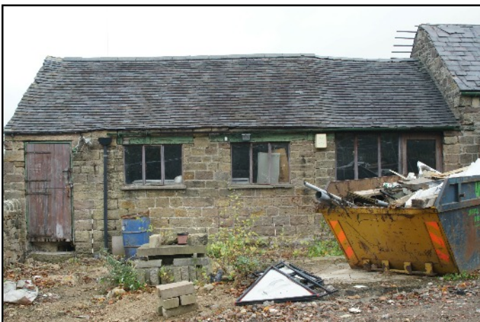
Plate 4: The south elevation of the West Section and Central Section, viewed looking north.
