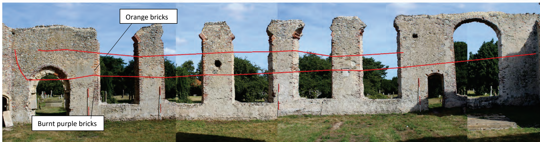
Plate 13. The internal face of the north aisle north wall showing the changes in build identified in the change of bricks
