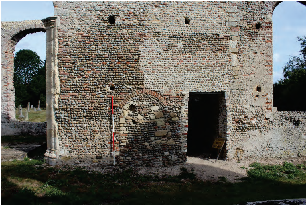
Plate 21 Interior of the north chancel with blocked and current entrances in to the Sacristy, following consolidation
