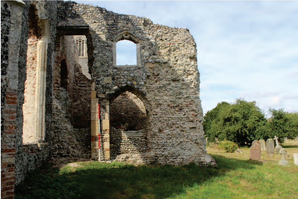
Plate 15. The exterior of the east wall of the north aisle, the elongated opening is the collapsed remains of a spiral stair. The windows light the ground and first floor rooms of the Sacristy. The limestone quoins behind the scale are all part of a modern repair.
