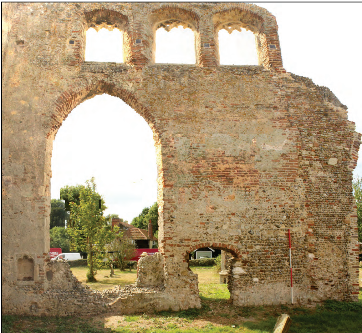
Plate 6. South wall of the chancel. The vertical joint where the chancel was connected to the nave can be seen to the right of the 2m scale. Above the priest door the wall face is composed almost entirely in brick a phenomenon which was not seen elsewhere and which contrasts with the nave and base of the chancel wall. The dropped sill at the base of the large window is thought to be a sedilia, whilst the priest door has been narrowed by building up the left jamb, the current ground level is c.0.5m above the medieval floor level.
