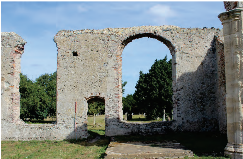
Plate 12. Area of the chapel at the north aisle, showing the large window and priest door. The socket, the possible location of a screen, can be seen near the top of the wall (above the scale).
