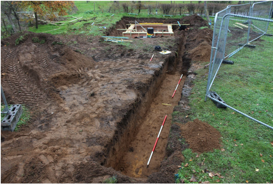
Plate 4. The arch drain trench was west of the site of the new WC (seen in the background). The arch drain trench was 7m long and 1m wide, increasing in depth from 600mm to 850mm, east to west. The scales are 2m long.
