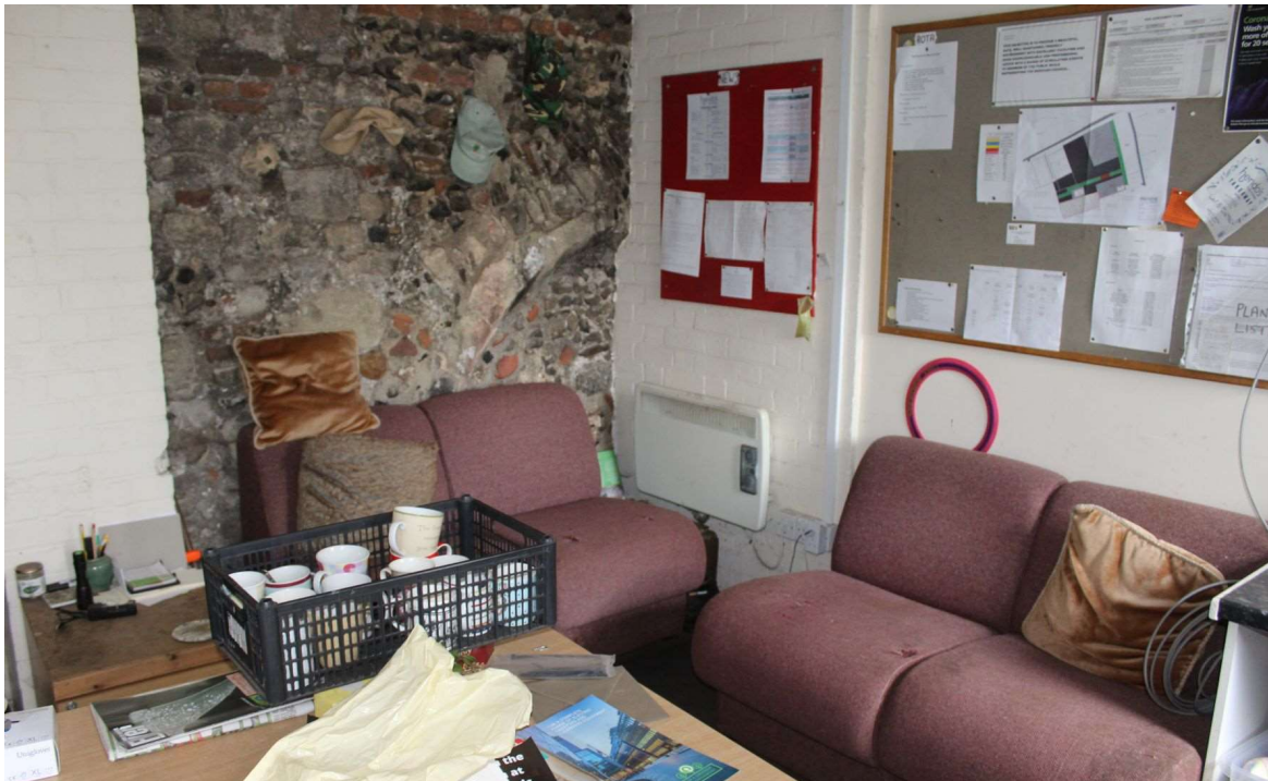
Plate 3. A blocked door in the rear wall of the gardener's mess room. The lower half has been buried by the rise in ground level and the top of the door is now only 1.2m from floor.
