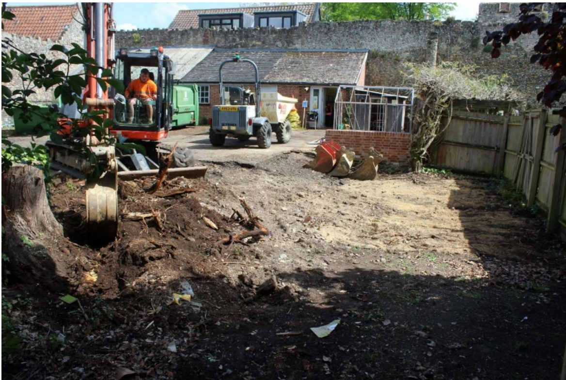
Plate 7. Area 3 the site of the Efford bed during the grubbing out of the trees and prior to excavation. The location was a soft-dig area beyond the edge of the tarmac yard and low-lying, where the ground fell away to the level of the adjacent garden, which is 300-400mm lower
