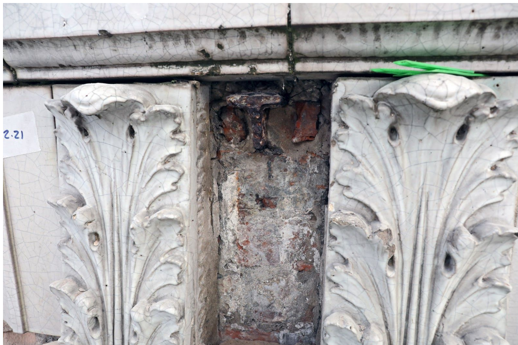
Figure 6 Canopy mounting location between two acanthus brackets, with the broken T-section joist visible at the top following the removal of the white-painted concrete.
