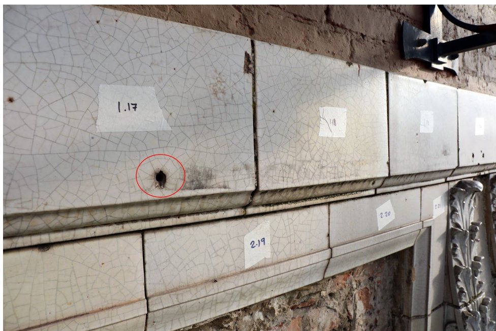
Figure 8 One of the small holes (highlighted in red) drilled into the top line of faience tiles as part of a canopy mount.
