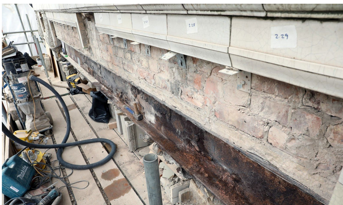
Figure 2 Removal of the faience pieces revealed the earlier brickwork behind, which is supported on a course of masonry sitting on a steel I-beam lintel.
