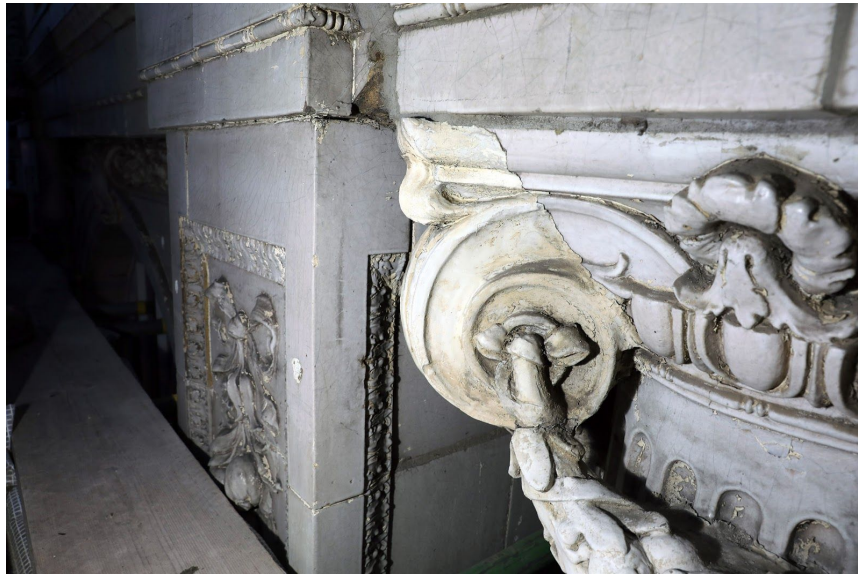
Figure 9 C20th repair to the left volute of the composite capital (6.5).
