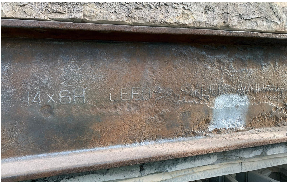
Figure 10 Visible lettering on the face of the Steel I-beam following cleaning. Corrosion from water ingress has deteriorated the beam and reduced its legibility to the right.
