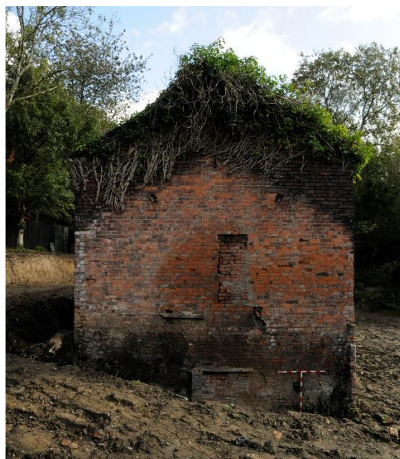
Figure 9 The west gable elevation with blocked opening and scar of former roof line
