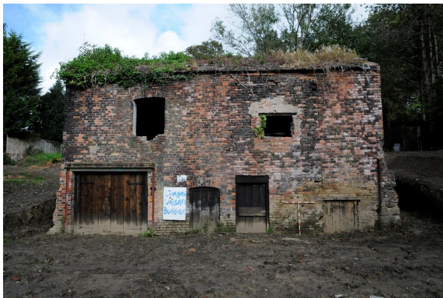
Figure 8 The south elevation of the barn with various blockings and with vertical joins at east side
