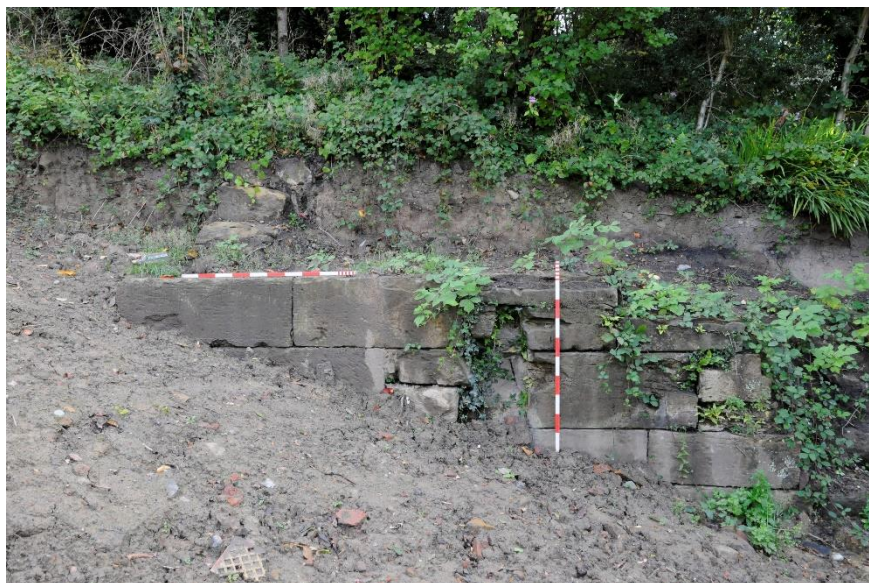
Figure 16 View of wall or revetment located at the east side of the site
