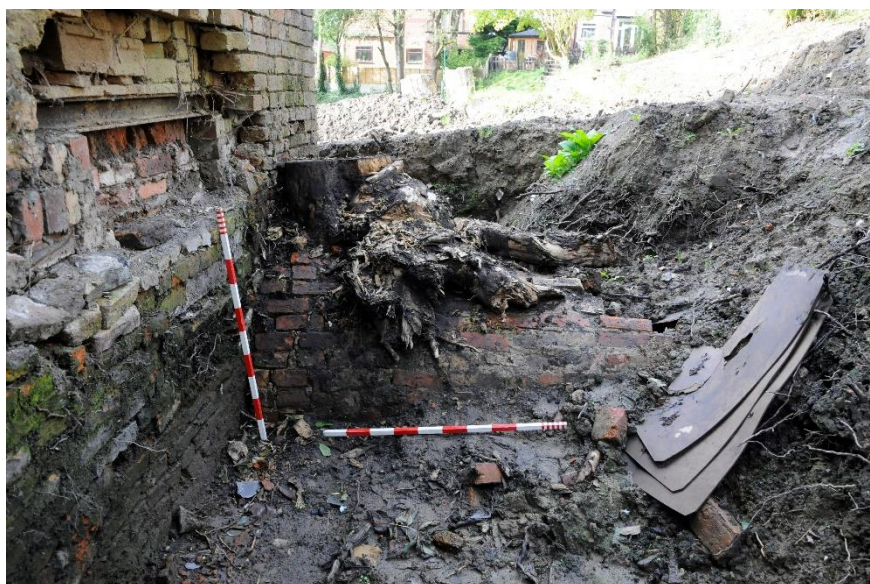
Figure 11 The arched flue or culvert on the north side of the building
