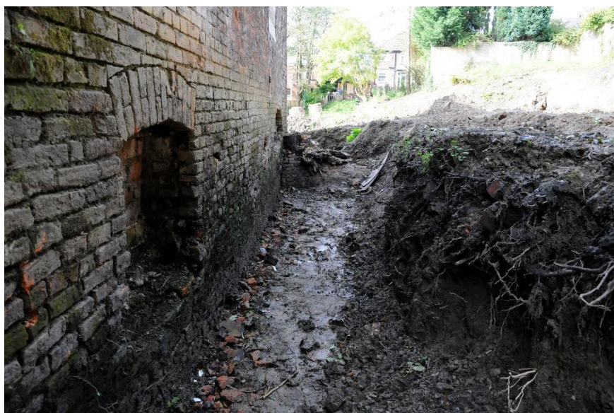
Figure 13 View of the trench and embankment at the north side of the building
