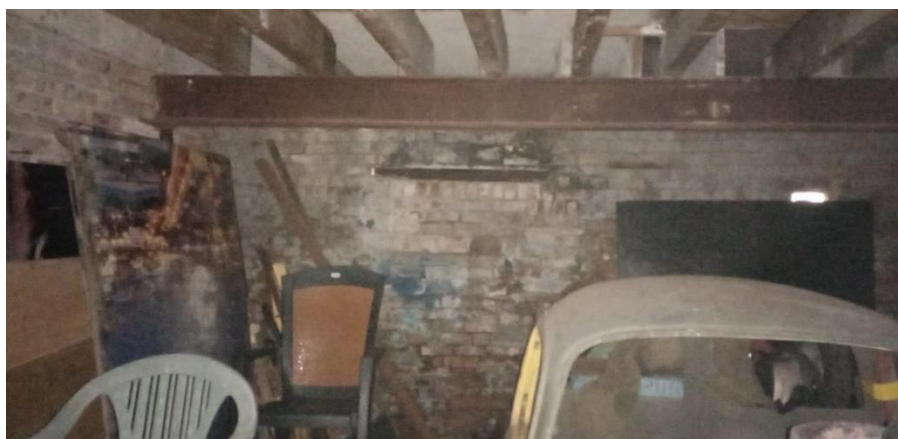
Figure 17 View at ground level showing an internal partition with modern RSJ supporting joists
