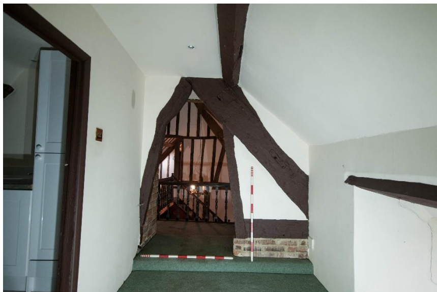
Figure 46 Room F4, looking south. Showing timber partition with inserted opening. Note truncated tie beam
