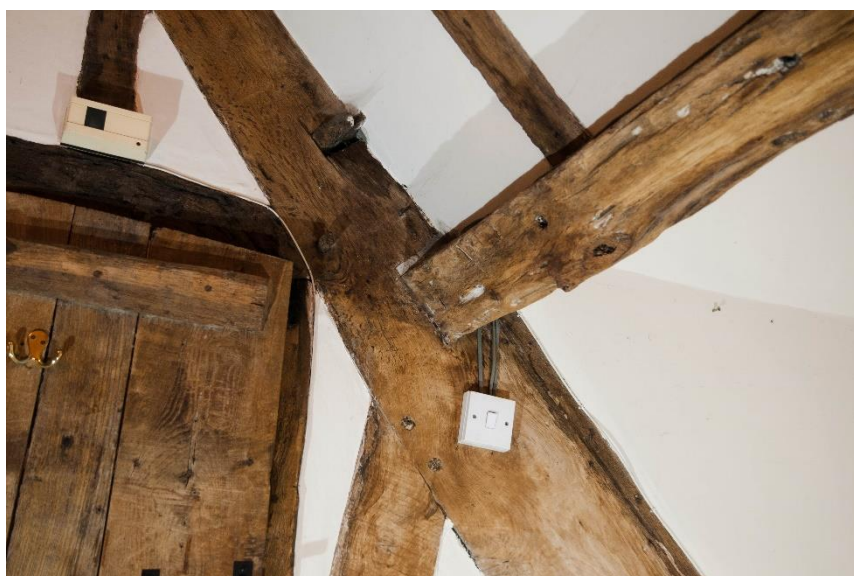
Figure 39 Room F2, detail of east side of partition, showing purlin in situ
