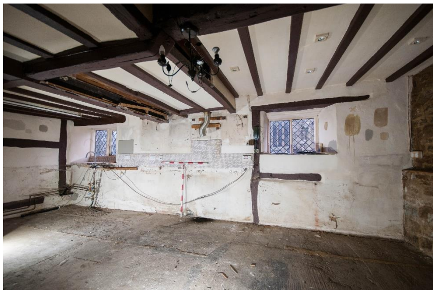
Figure 31 Room G4, the west wall; the blocked paired openings are positioned between the windows
