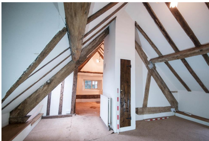
Figure 41 Room F2, looking south and showing modern chimney; note truncated tie beam
