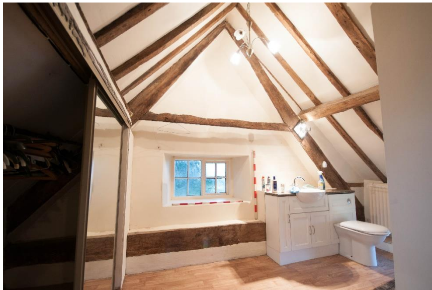
Figure 44 Room F3, looking south and showing roof truss partly embedded in the south wall
