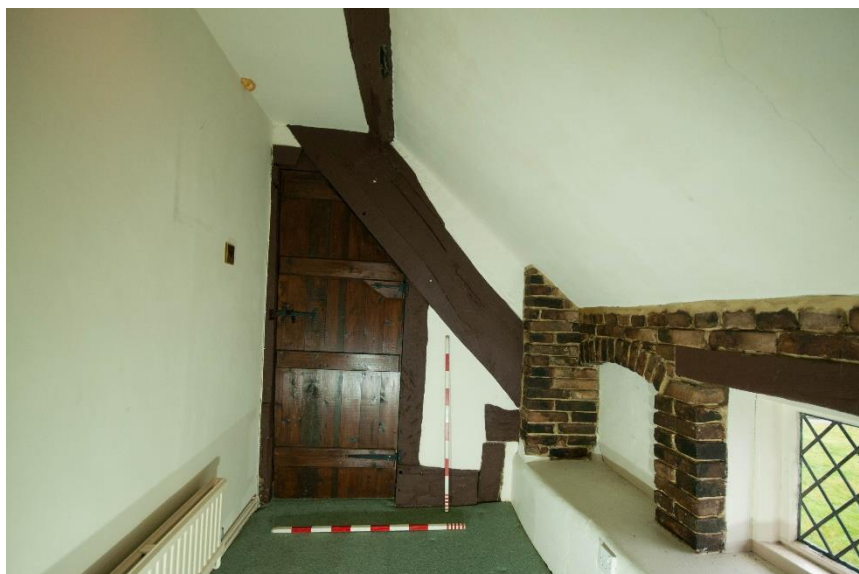
Figure 47 Room F5, looking south. Showing timber partition with inserted door. Note truncated tie beam
