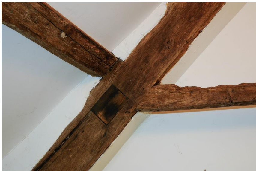
Figure 38 Room F2, detail of west side of partition showing moved purlin, and join to collar
