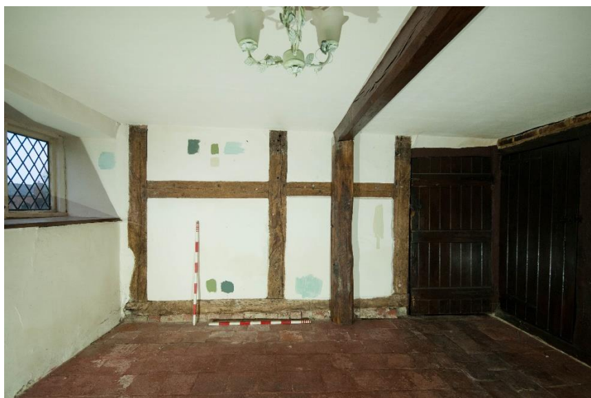
Figure 27 The north wall of Room G3; note the modern beam supported on a free standing post
