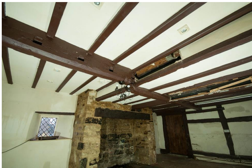
Figure 32 Room G4, view of the spine beam with defunct joist slot; note the change in ceiling level marking the position of an RSJ
