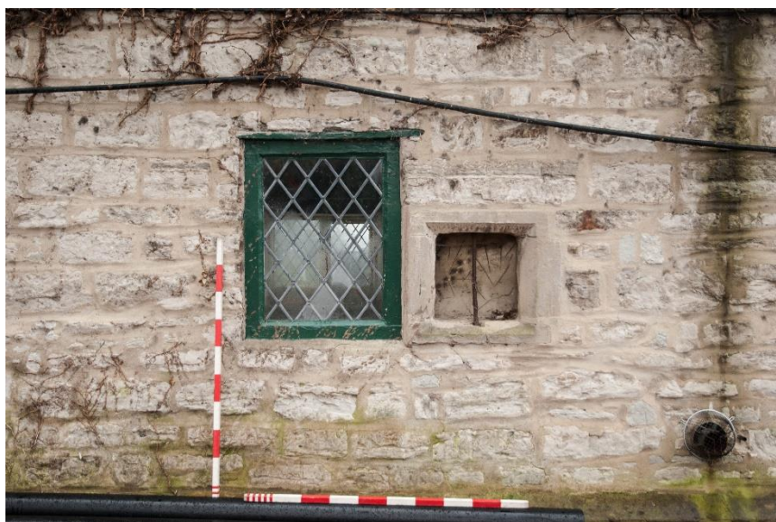
Figure 17 Detail of windows on the east elevation, showing the small blocked opening
