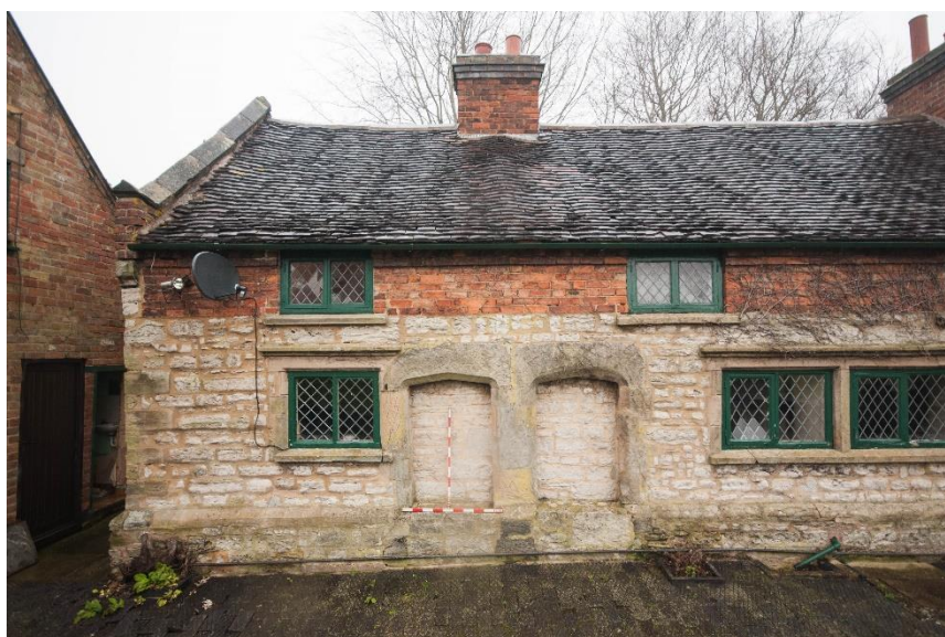
Figure 7 The north end of the west elevation with blocked paired doorways and modern windows in the historic openings
