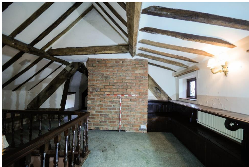
Figure 33 Room F1, looking north and showing railings to the galleried walkway and modern brick chimney;
