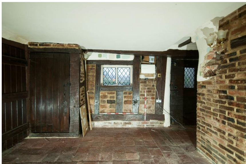
Figure 26 Room G3, looking east, showing the modern rebuilding of the wall
