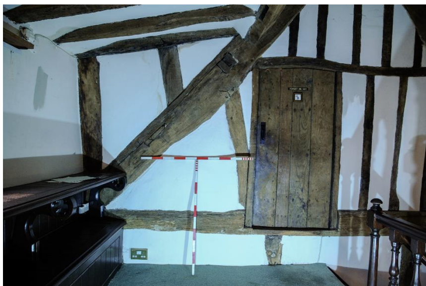
Figure 35 Room F1, historic partition with inserted door. Also showing modern dormer framing
