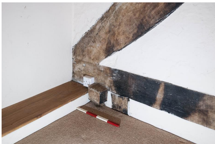
Figure 37 Room F2, detail of the truss / tie beam join with remnant wall plate
