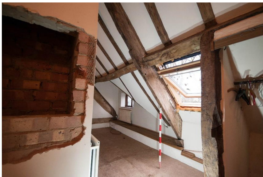
Figure 43 Room F3, looking north to F2, showing intervening partition. Note modern chimney to left
