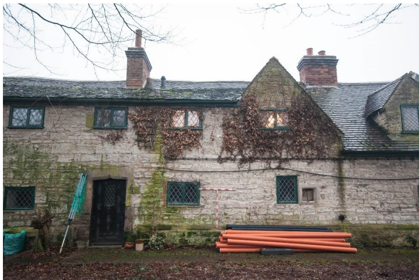
Figure 16 View of the east elevation showing the 1970s dormer overlying the earlier wall level
