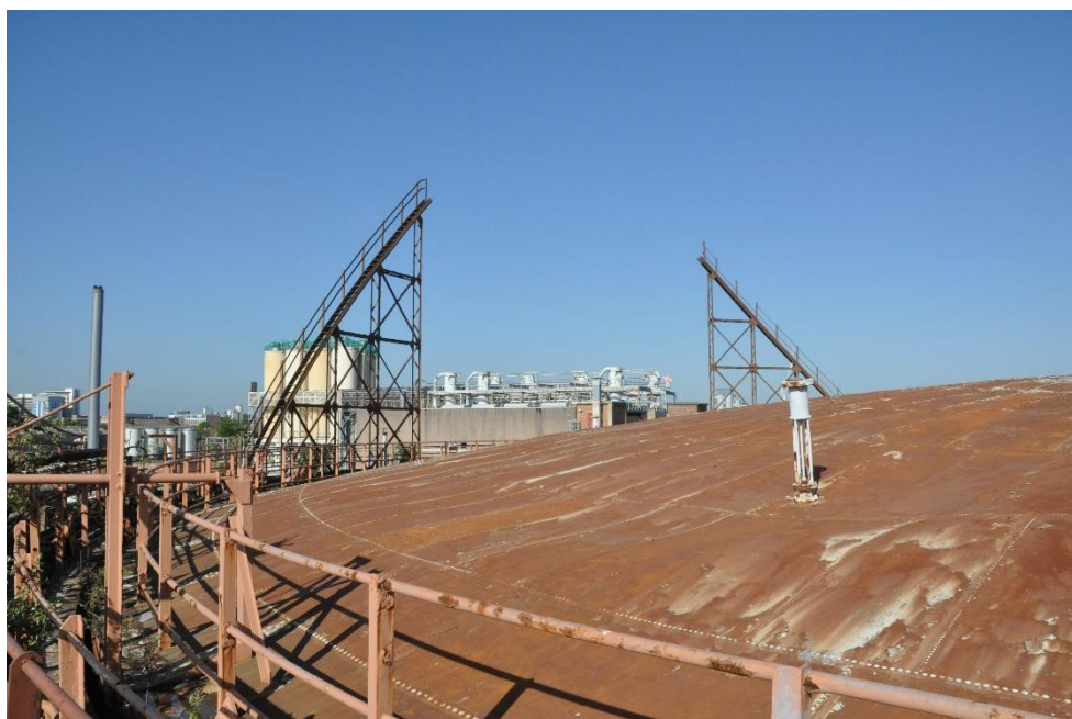
Figure 11: View of the crown, looking south-west and showing maglock knock-off arms and a hydrostatic tank.
