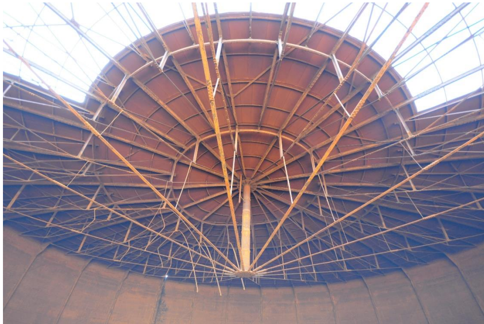
Figure 15 The crown frame and central pipe.
