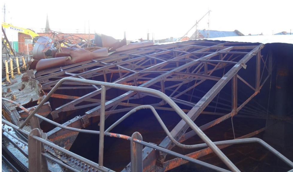
Figure 1 Gasholder 1, view of the crown frame, showing trusses spanning between the central pipe and gusset plates attached to vertical stiffeners
