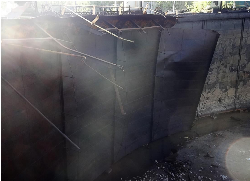
Figure 7 Gasholder 2, view of the inner lift showing the top curb and vertical stiffeners
