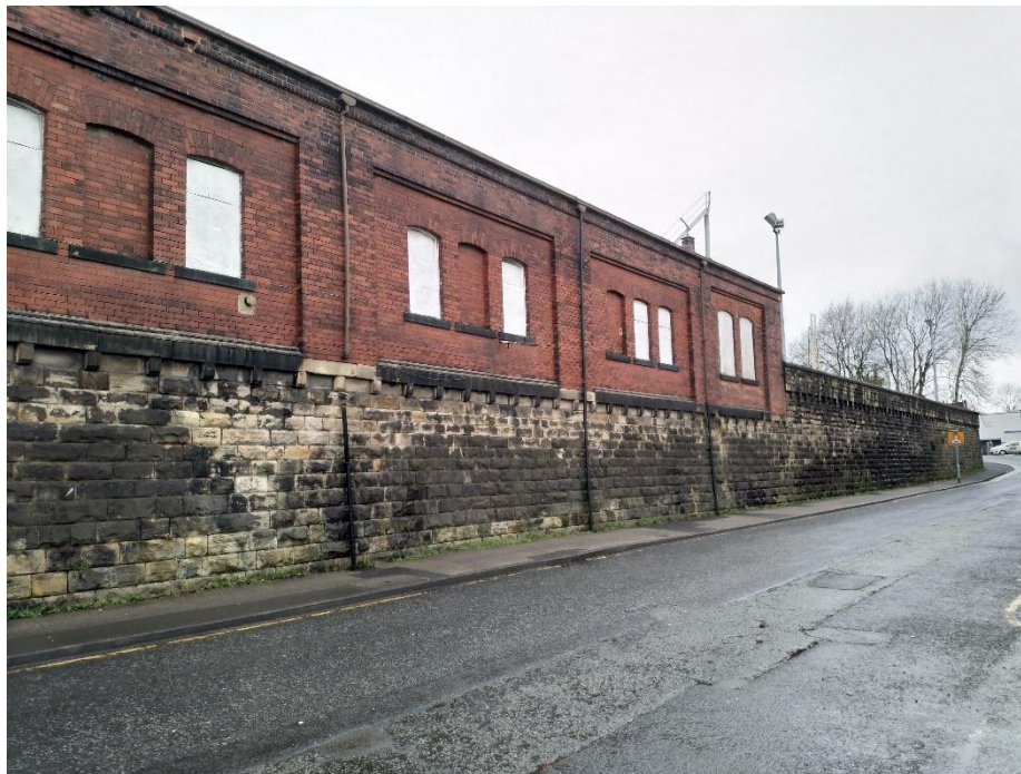
Figure 28: View of the laboratory building and retaining wall on the west side of Victoria Road.
