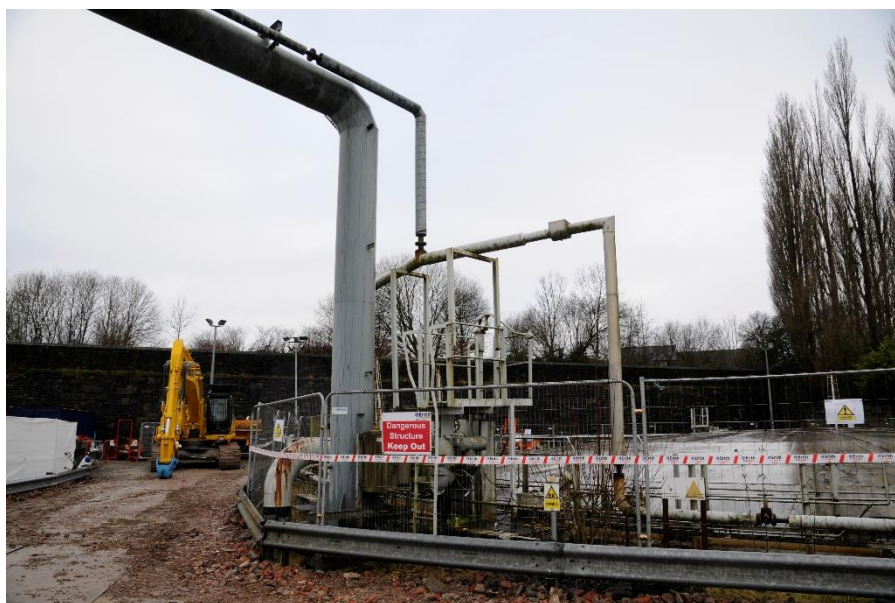
Figure 8: Gas mains and anti-freezes joining the south side of Gasholder 1.
