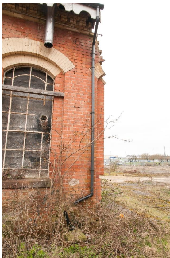
Figure 18 The west end of the north elevation showing remains of former window
