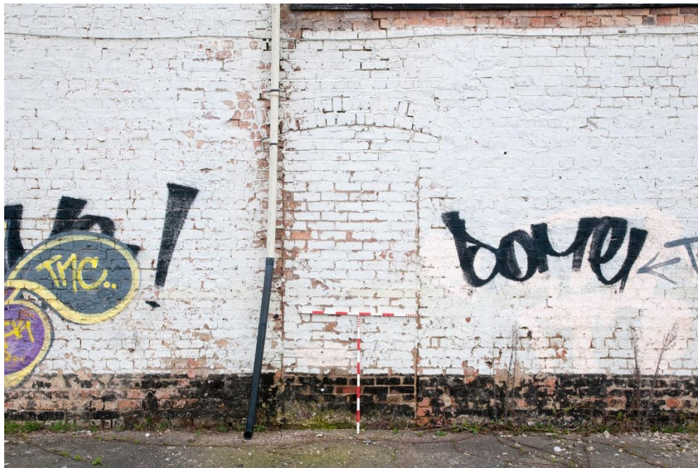
Figure 3 Detail of blocked door on the south elevation
