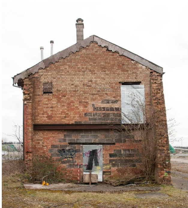
Figure 19 The repaired west elevation with remains of wall returns; showing blocked doors and inserted RSJ
