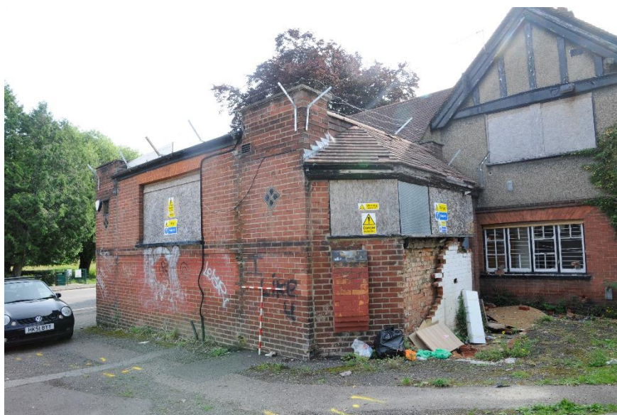
Figure 5 General view of the single storey block and bay window, looking north-east
