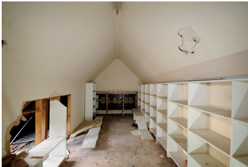
Figure 37 Room F6, looking north, showing the construction of the stud partition wall
