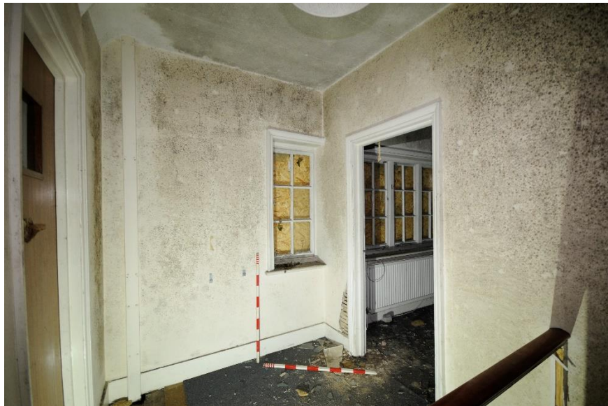
Figure 30 The north side of the first floor landing showing intersection of window and partition wall
