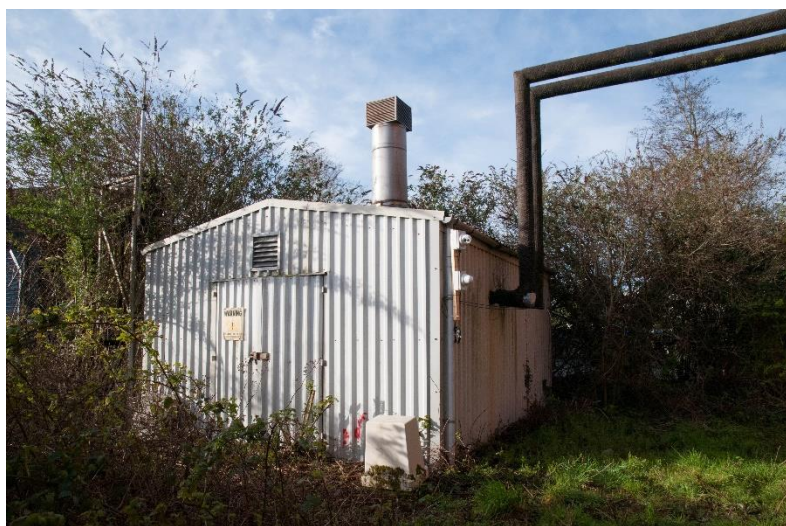
Figure 28 The modern boiler room with lagged pipes
