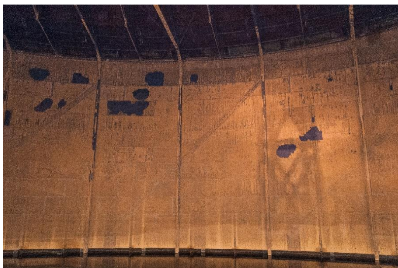
Figure 22 View of the inside face of the crown lift, showing vertical stiffeners and attachments for spiral rails
