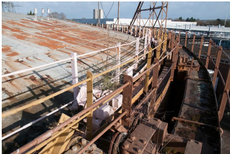
Figure 7 View of the crown, lifts and walkway, looking north from the east side of the gasholder
