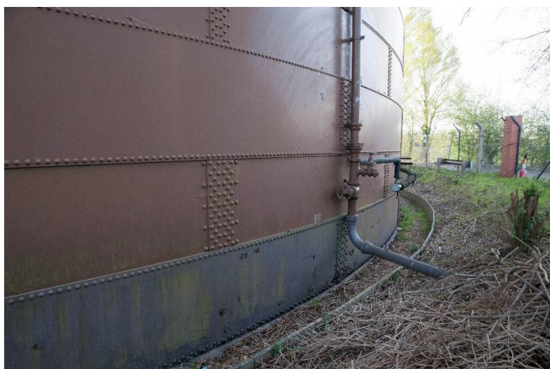
Figure 4 View of the tank and anti-freeze pipes, showing the base of gasholder and embankment
