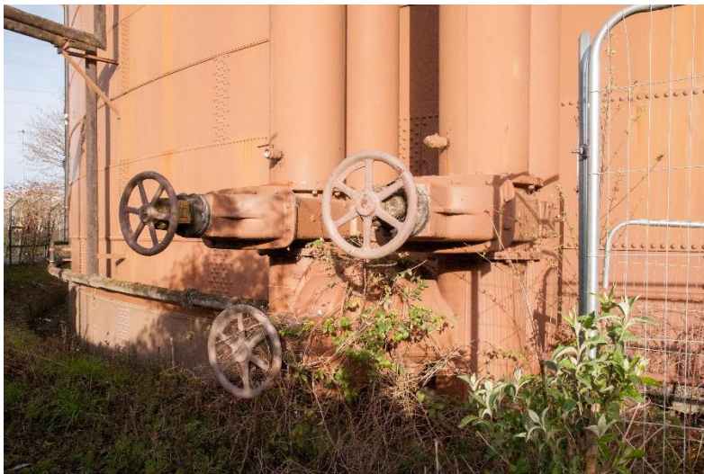
Figure 13 Flow valves attached to the inlet / outlet pipes
