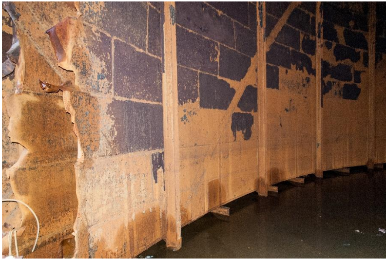
Figure 23 View of inside face of lifts, showing rest blocks and vertical stiffeners
