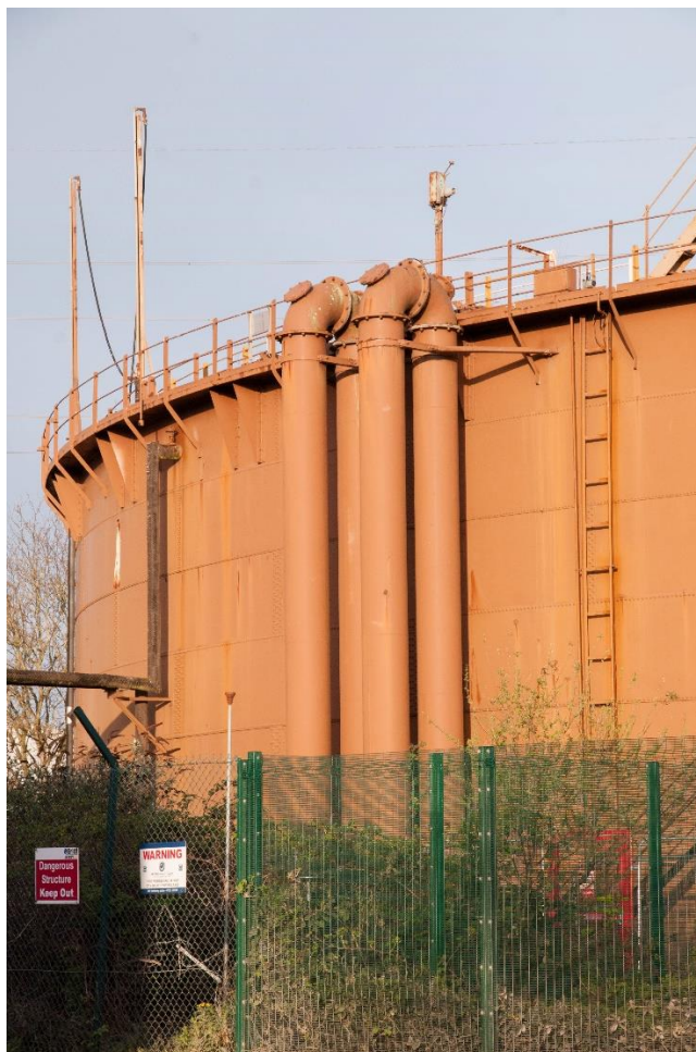
Figure 12 The inlet / outlet pipes
