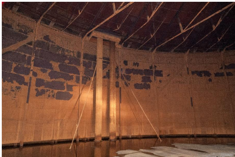
Figure 20 View of the inlet and outlet pipes
