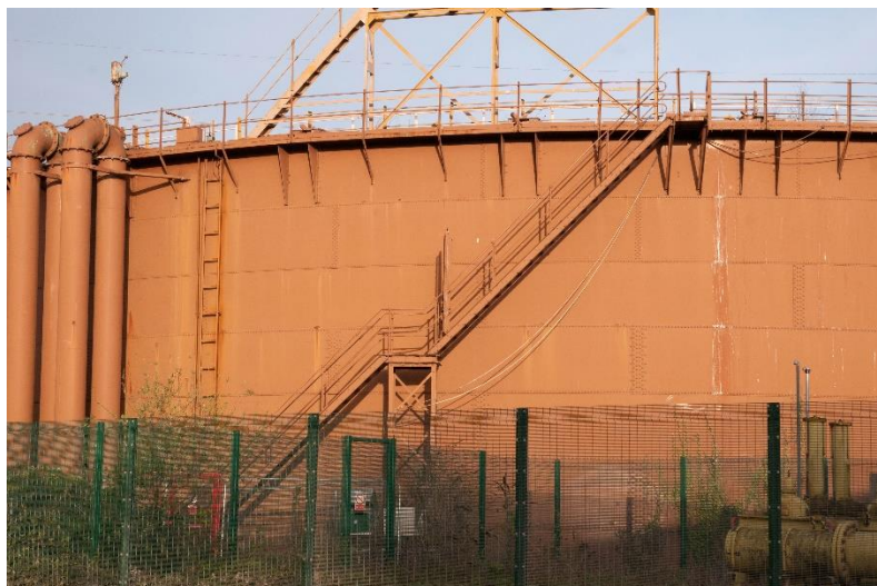
Figure 5 View of the tank stair with inlet / outlet pipes at the left of image
