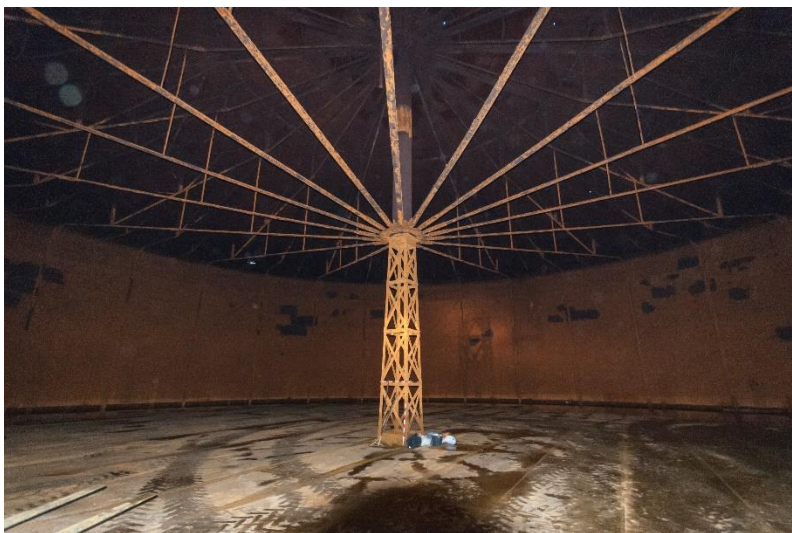
Figure 14 General view of the interior of the gasholder showing crown frame and support
