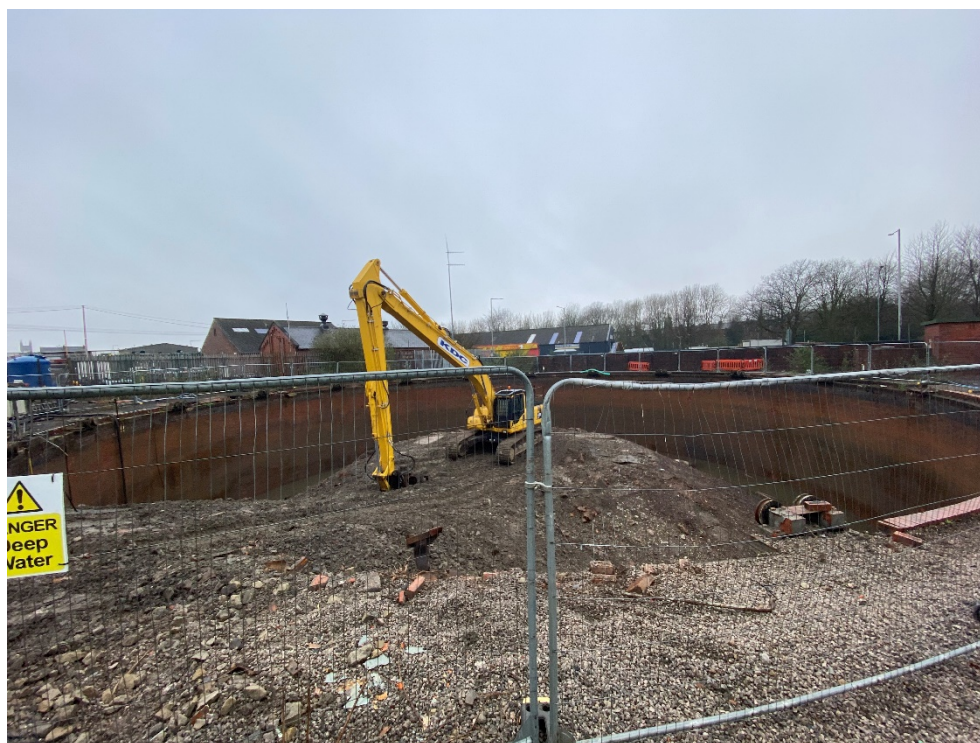
Figure 1: View of Gasholder 1 at time of survey with brick tank and dumping visible.
