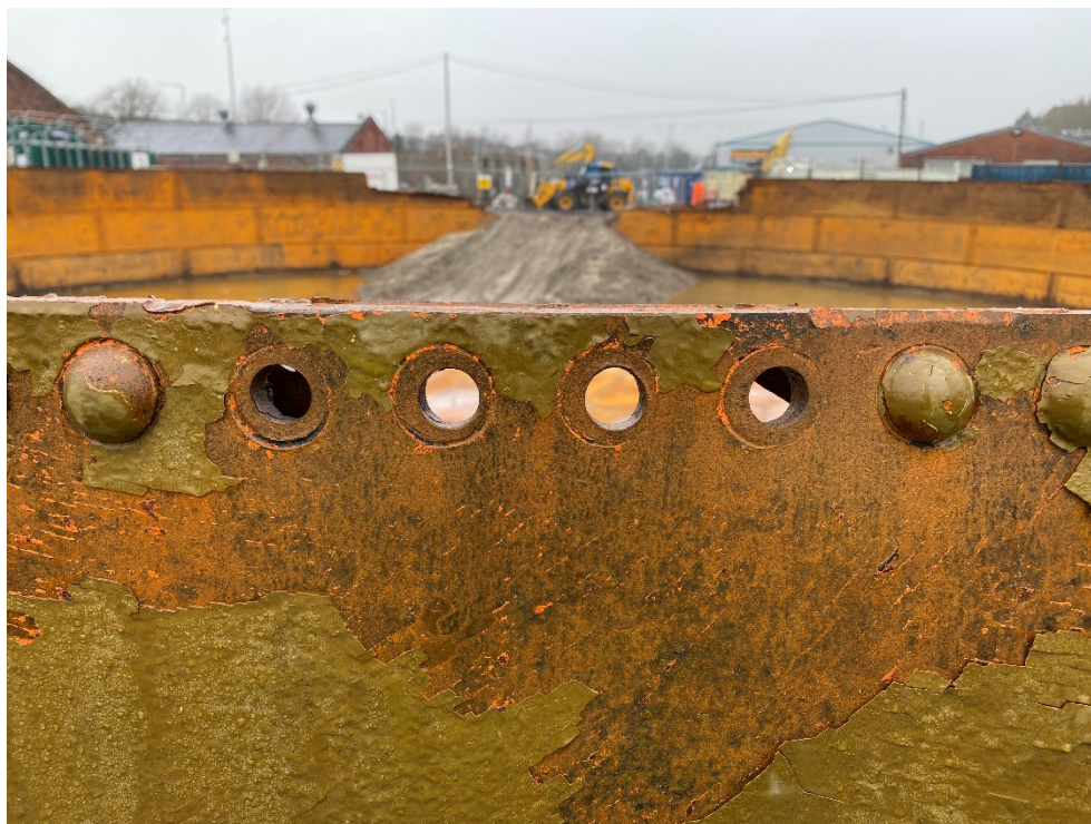
Figure 8: Detail of rivets in the steel tank sheeting.
