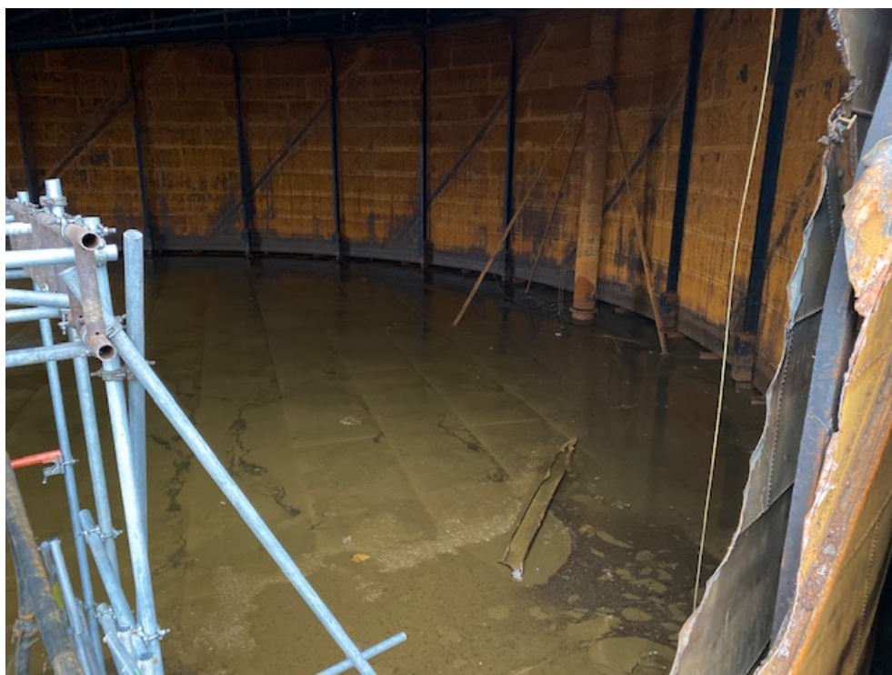
Figure 11: Interior of Gasholder 2 innermost lift. Inlet/outlet pipe visible.
