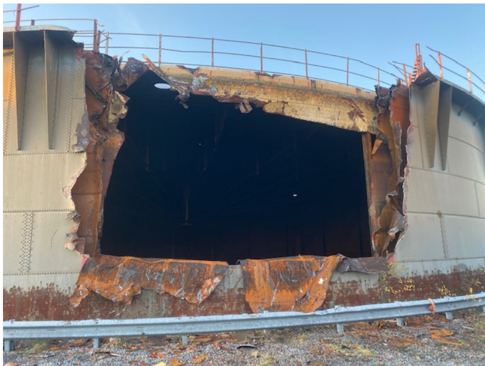
Figure 10: Demolition of Gasholder 2, crown frame visible inside innermost lift. Provided by demolitions contractor.
