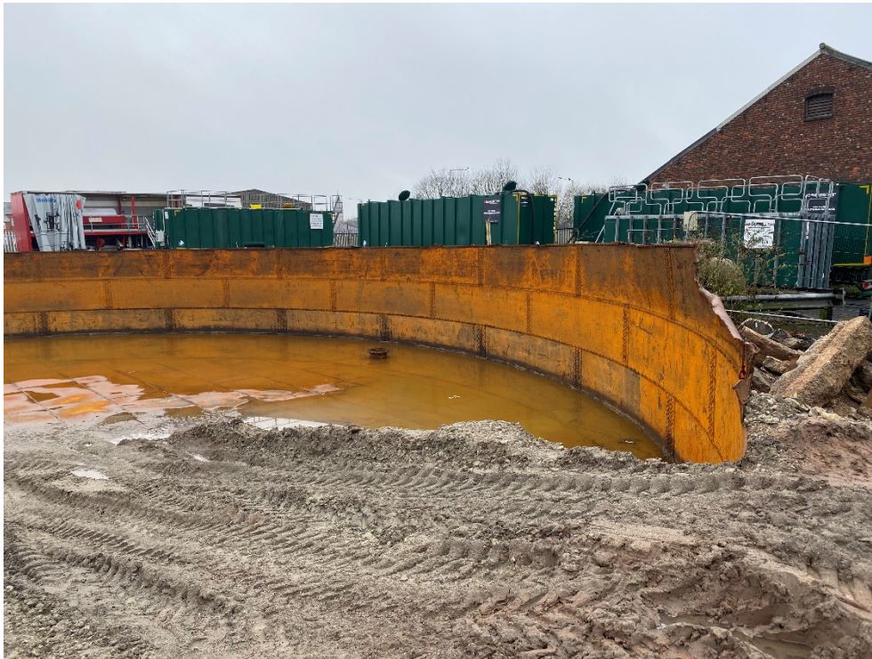
Figure 6: Extant lower courses of the tank at Gasholder 2. Base of inlet/outlet pipe visible.
