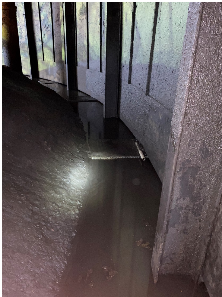
Figure 5: View of concrete rest pads within annulus of Gasholder 1. Provided by demolitions contractor.
