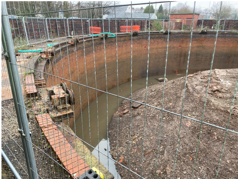
Figure 3: View of Gasholder 1 concrete and brick curb, roller carriages, brick tank, water filled annulus and dumping.
