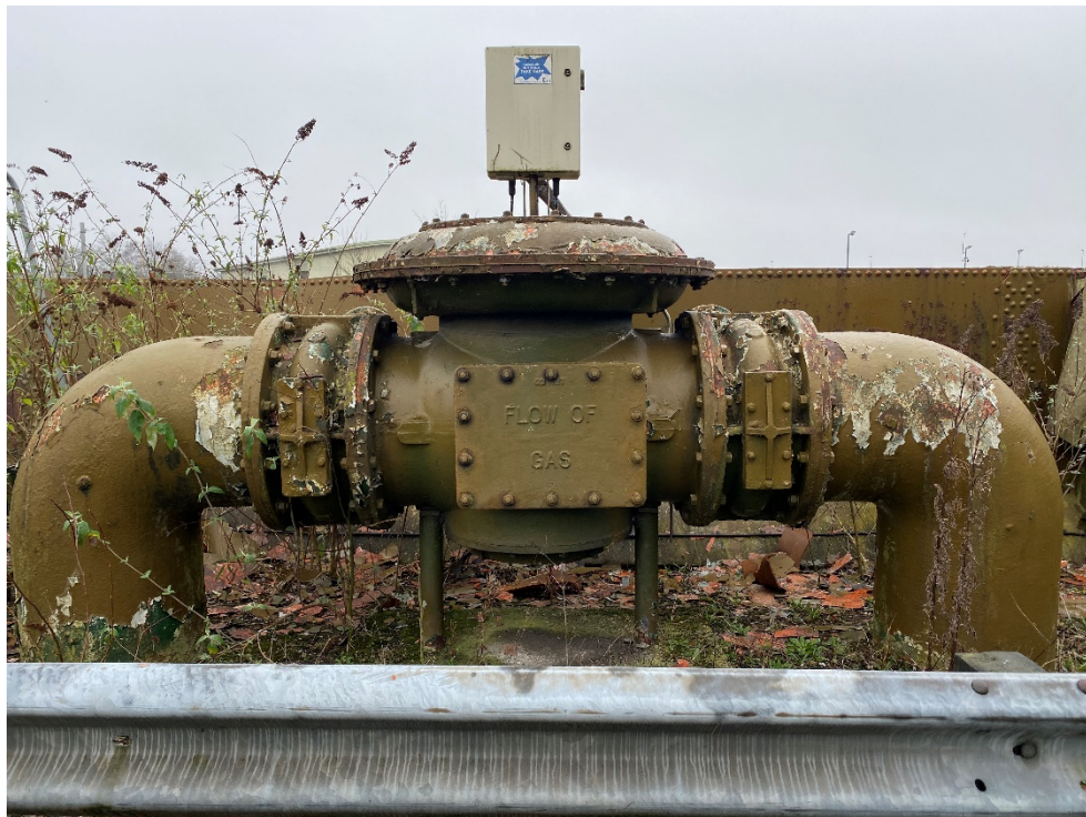
Figure 9 Flow Valve for Gasholder 2.
