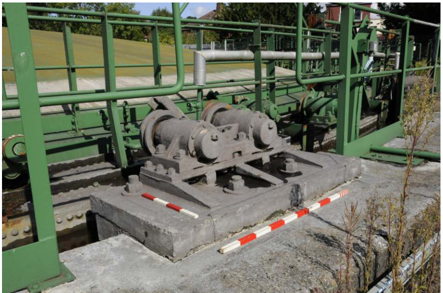
Example of the roller carriages Fig 34
