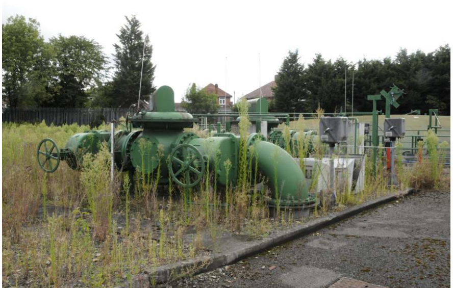
View of pipes and valves adjacent to Gasholders 1 and 2 Fig 40
