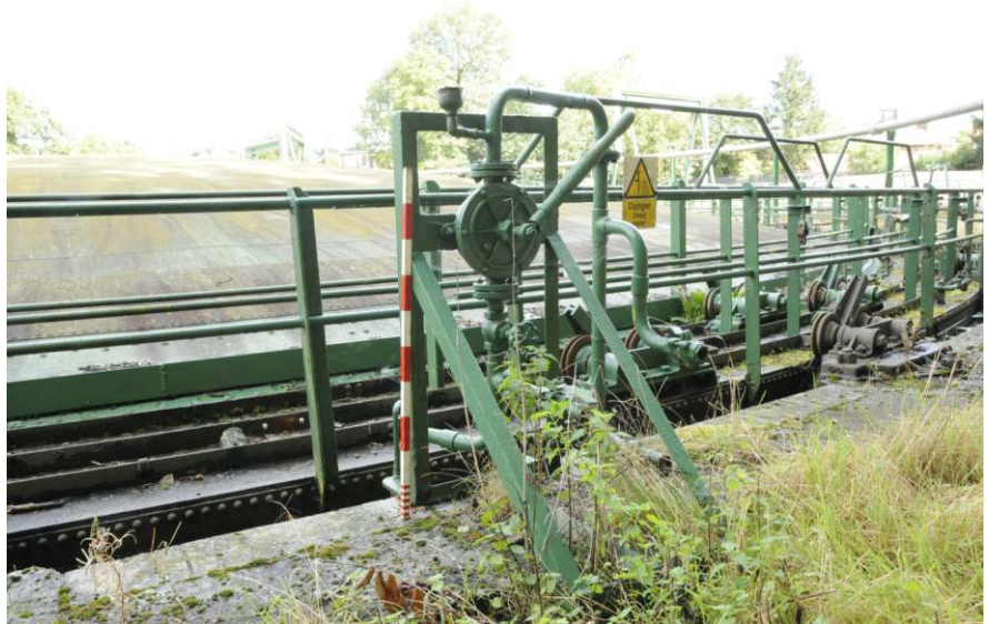
Manually operated overflow pipe valve Fig 24
