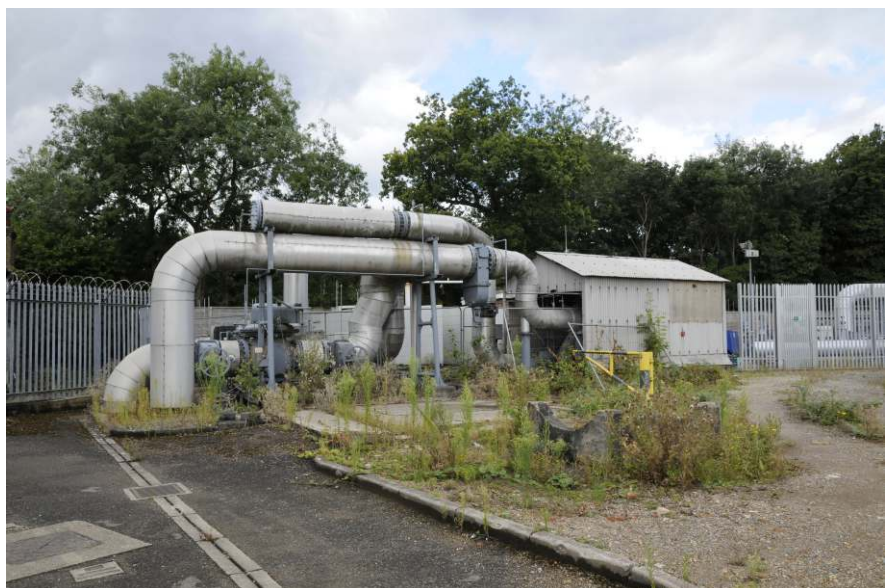
View towards PRS compound and pipes / valve house Fig 38
