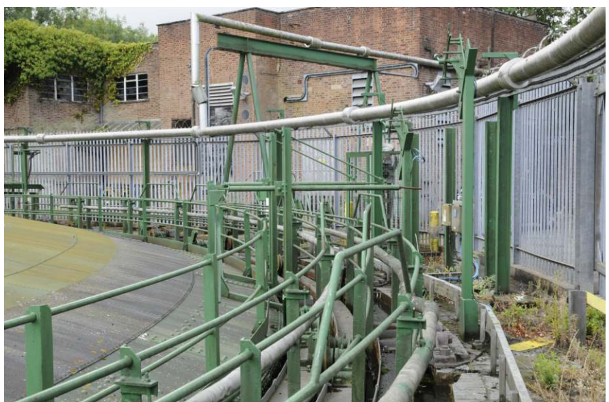
Elevated maglocks and lift knock-off arms, also showing lagged pipes to Booster House Fig 20
