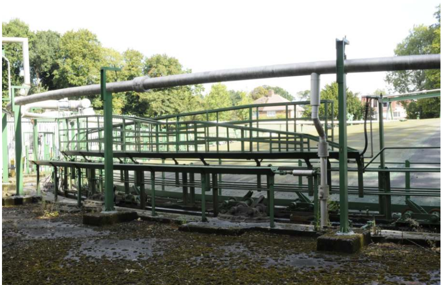
Pivoting steam pipe trays and overhead lagged pipes at the south of the gasholder Fig 23
