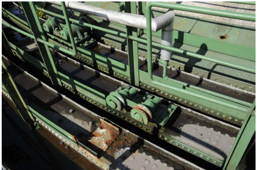
Detail of the lift grips, showing roller carriage and lagged pipe Fig 37
