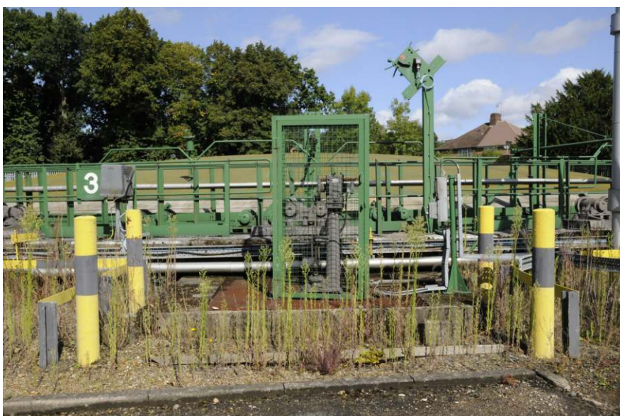
Dry-well and syphon pump at the south side of the gasholder Fig 29
