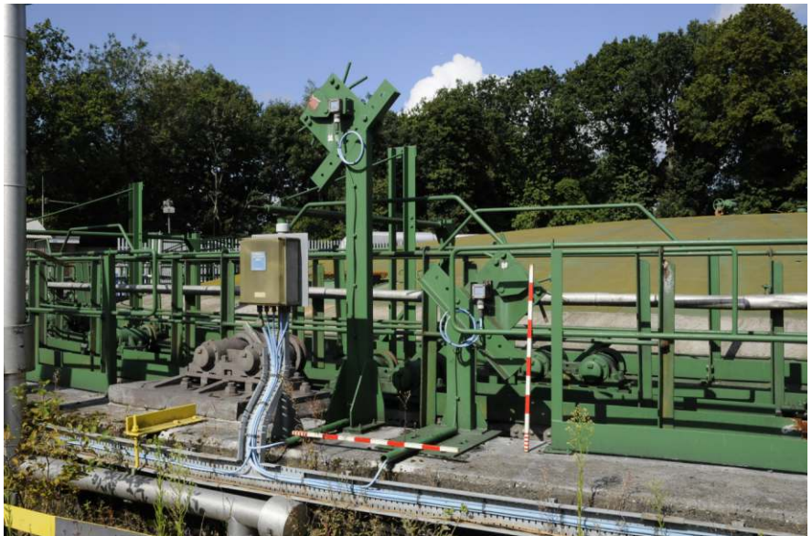
Detail of electric cables and maglocks Fig 30
