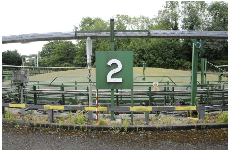
Detail of signage, also showing vehicle barrier and overhead cable tray Fig 19
