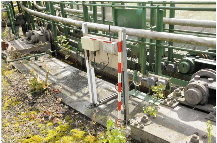
Electronic monitoring and telemetry and anti-freeze units Fig 15
