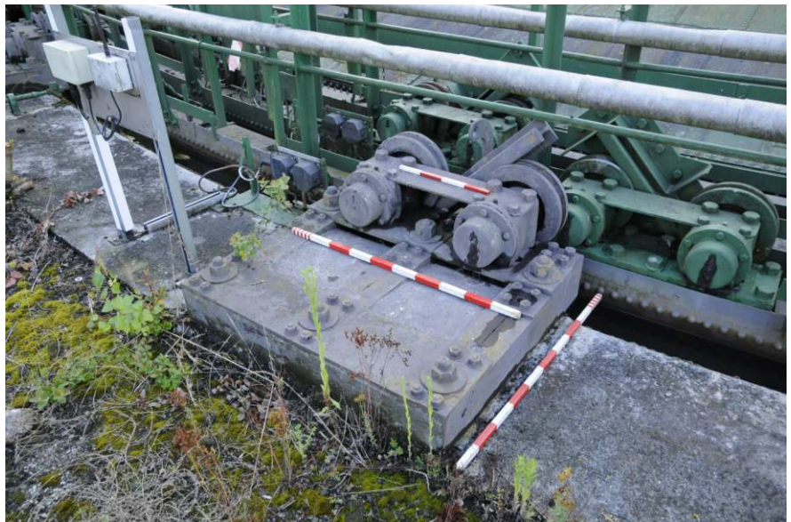
Example of the roller carriages Fig 16
