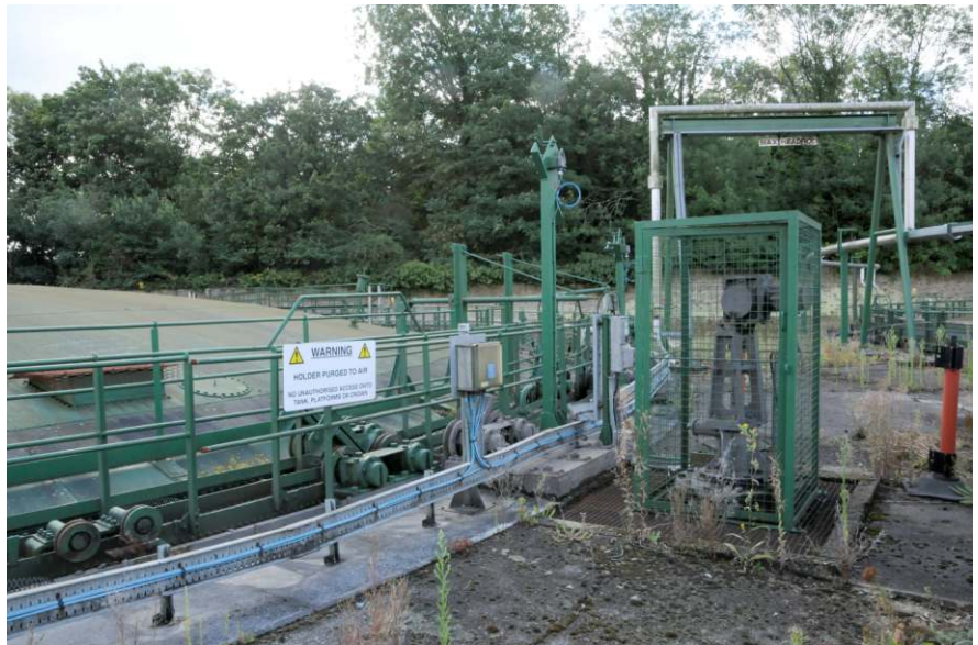
Dry well and syphon pump, as well as electrical cables at the east side of the gasholder Fig 12
