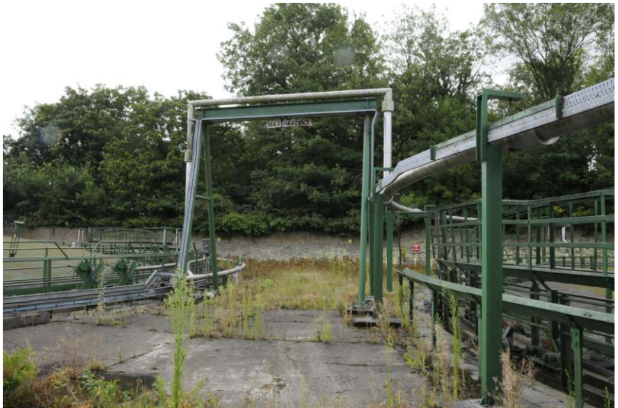
Overhead pipe and cable gantry between Gasholder 1 and 2 Fig 39
