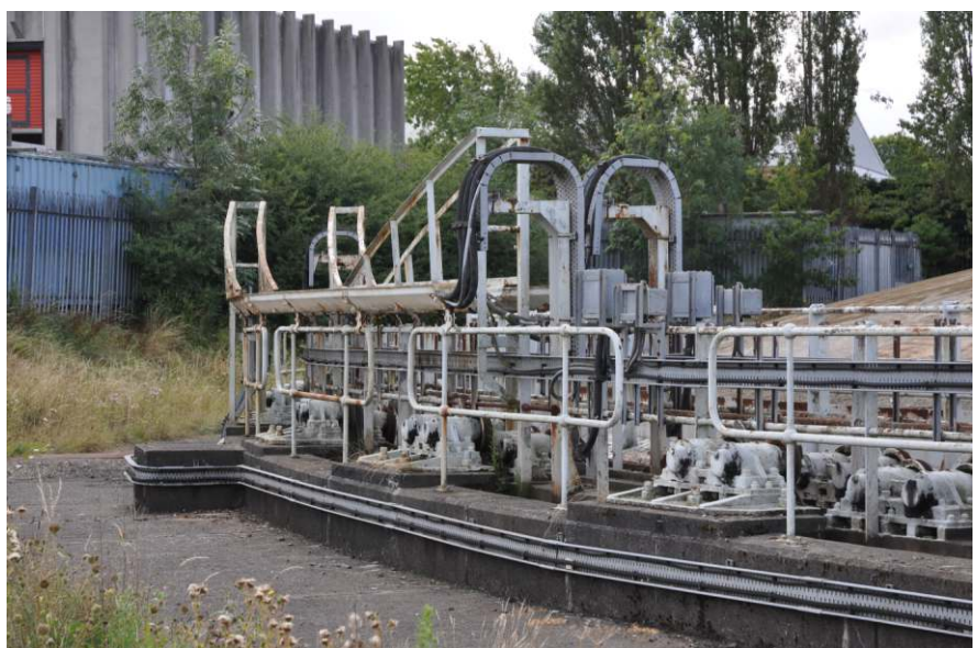
View of the pivoting cable trays Fig 19
