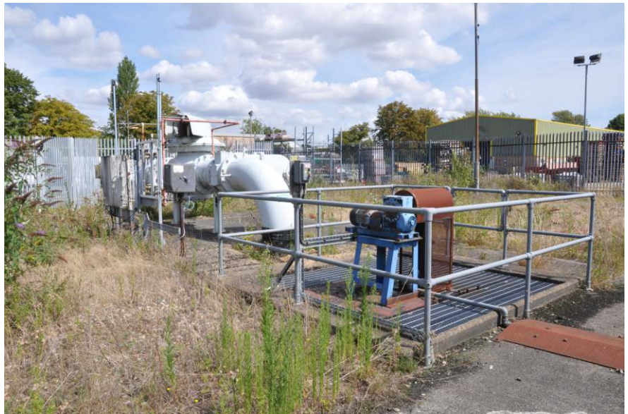
Dry well and pump with flow valves at the north side of the gasholder Fig 26
