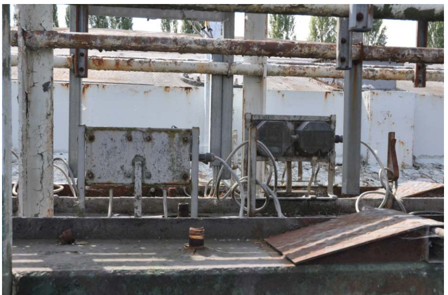
Example of the electrical anti-freeze fittings Fig 25
