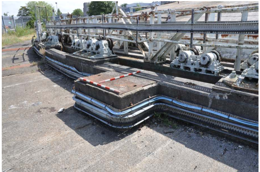
Detail of the raised kerb with well access. Note truncated stair Fig 20
