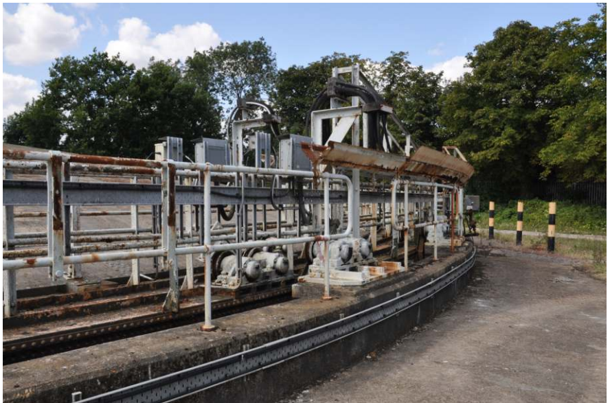
Pivoting cable trays at the north-east side of the tank Fig 8
