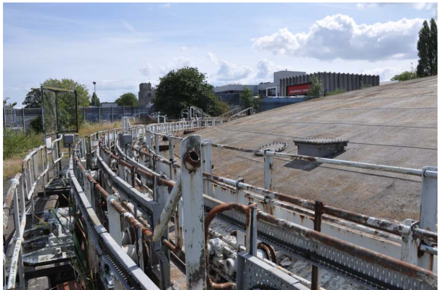
View of the lift handrails and crown with manholes; looking east Fig 21
