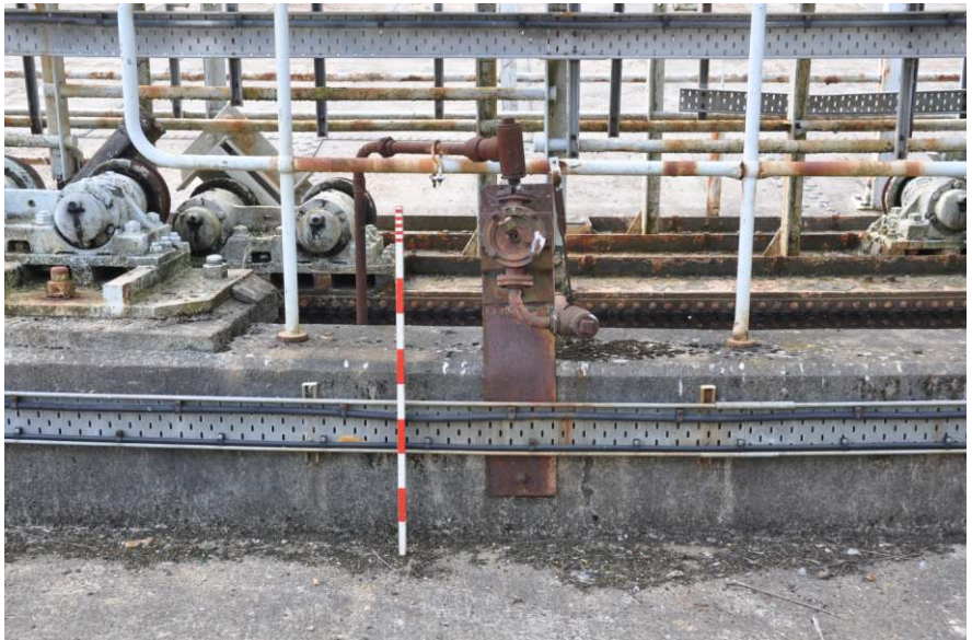
Overflow pipe and valve Fig 12
