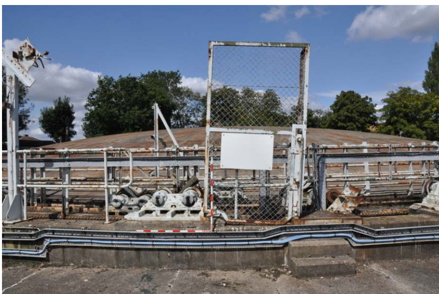
View of the raised tank kerb with stair and access barrier Fig 6
