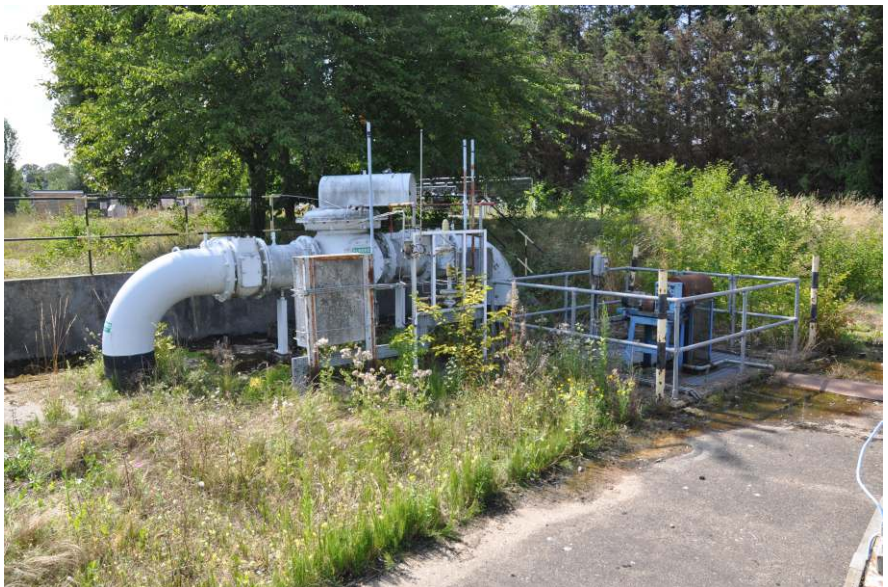
Dry well with pump and flow valves at the south of the gasholder Fig 9
