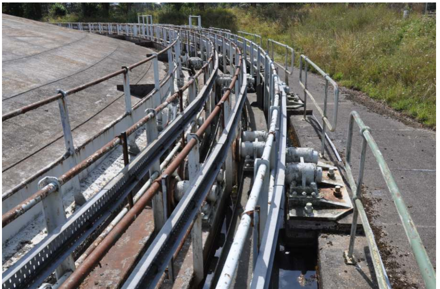
View of tank and lifts with handrails Fig 24
