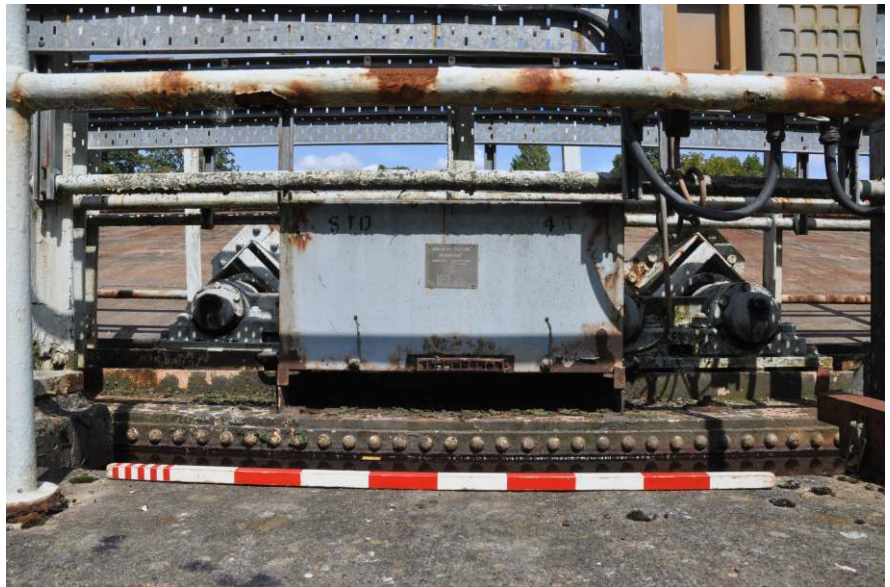
Example of the modular electrical anti-freeze units Fig 14
