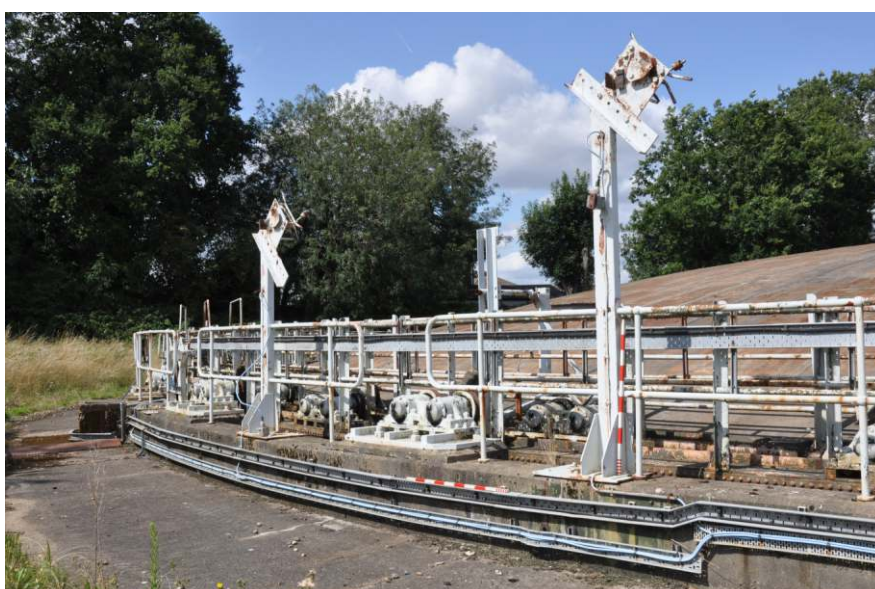
View of the elevated maglocks and knock-off arm Fig 7
