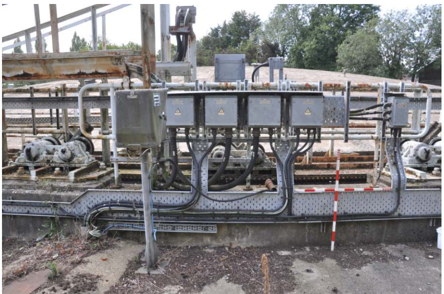
Electrical cables and controls Fig 13
