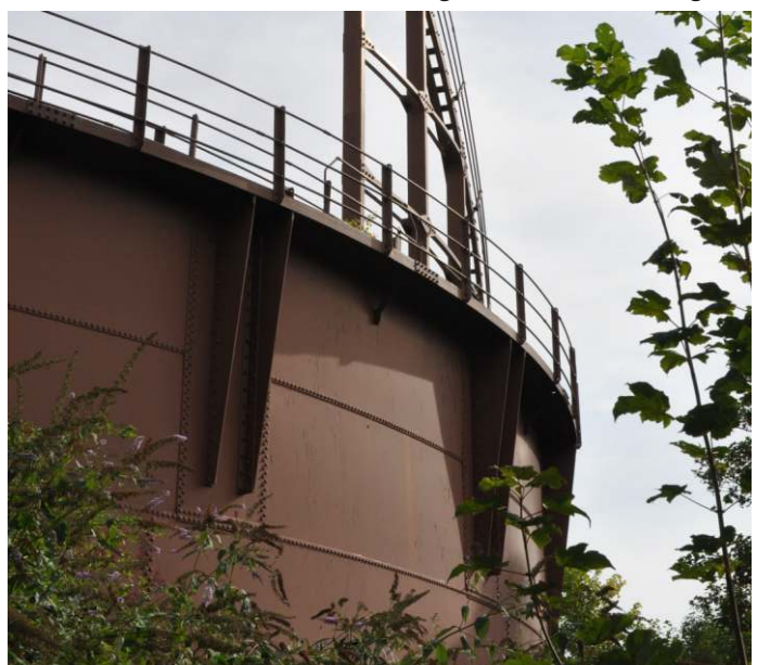
Detail of the tank and gussets Fig 19
