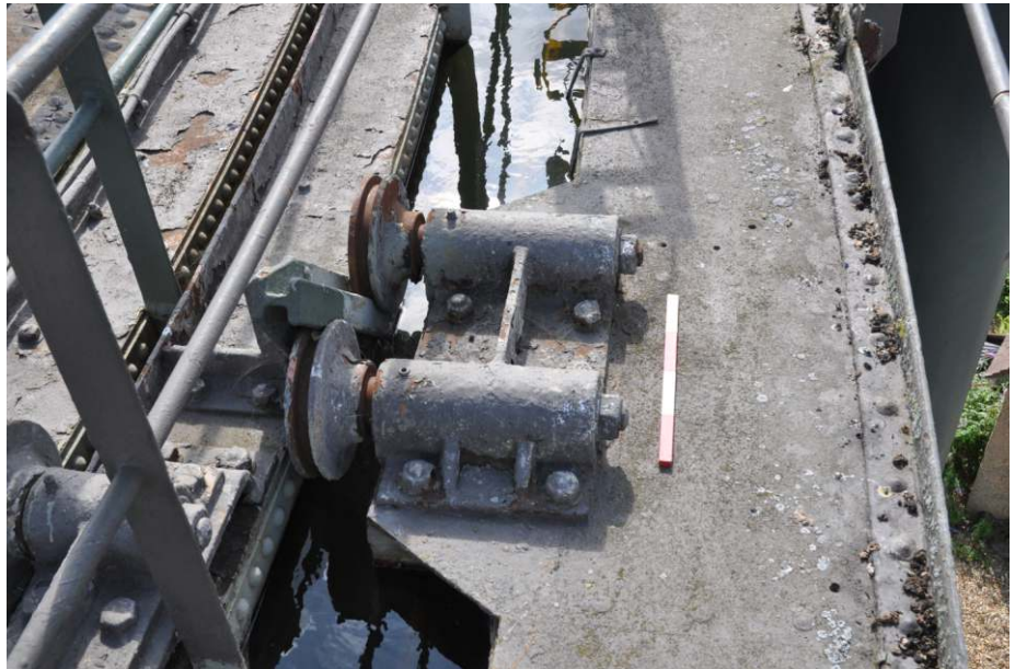
Example of the tank roller carriages Fig 15
