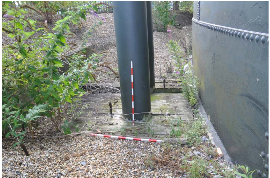
Redundant pipes and dry-well Fig 9
