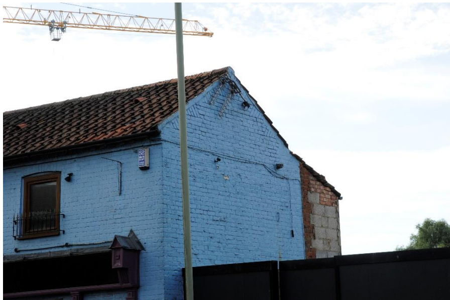
Figure 24 Detail of the west gable elevation with 'tumbled-in' bricks at the gable
