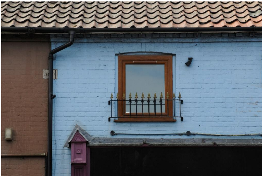
Figure 21 First floor window to No. 67. Note date stone of 1816 set behind the downpipe
