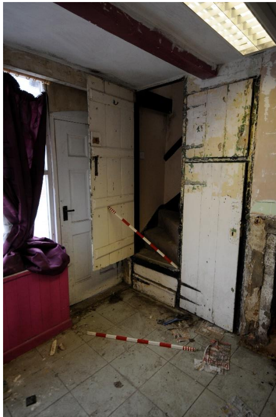
Figure 9 View of the stair access with door propped open. Note hinged bottom step below open door
