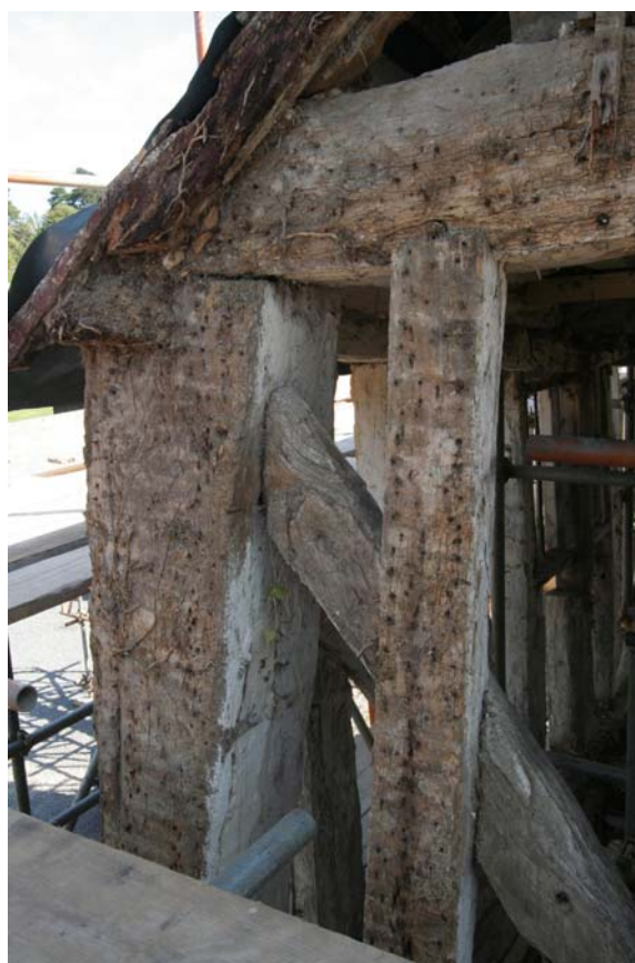
Plate 18: First floor exterior, north east corner (Showing plaster filled mortise in the white-washed face, below the diagonal brace)
