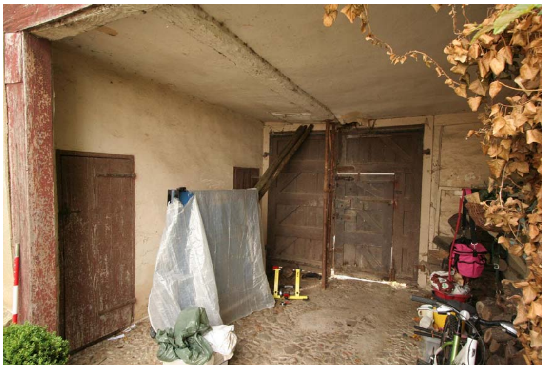
Plate 8: Ground floor interior (General view of the interior looking towards the north east)
