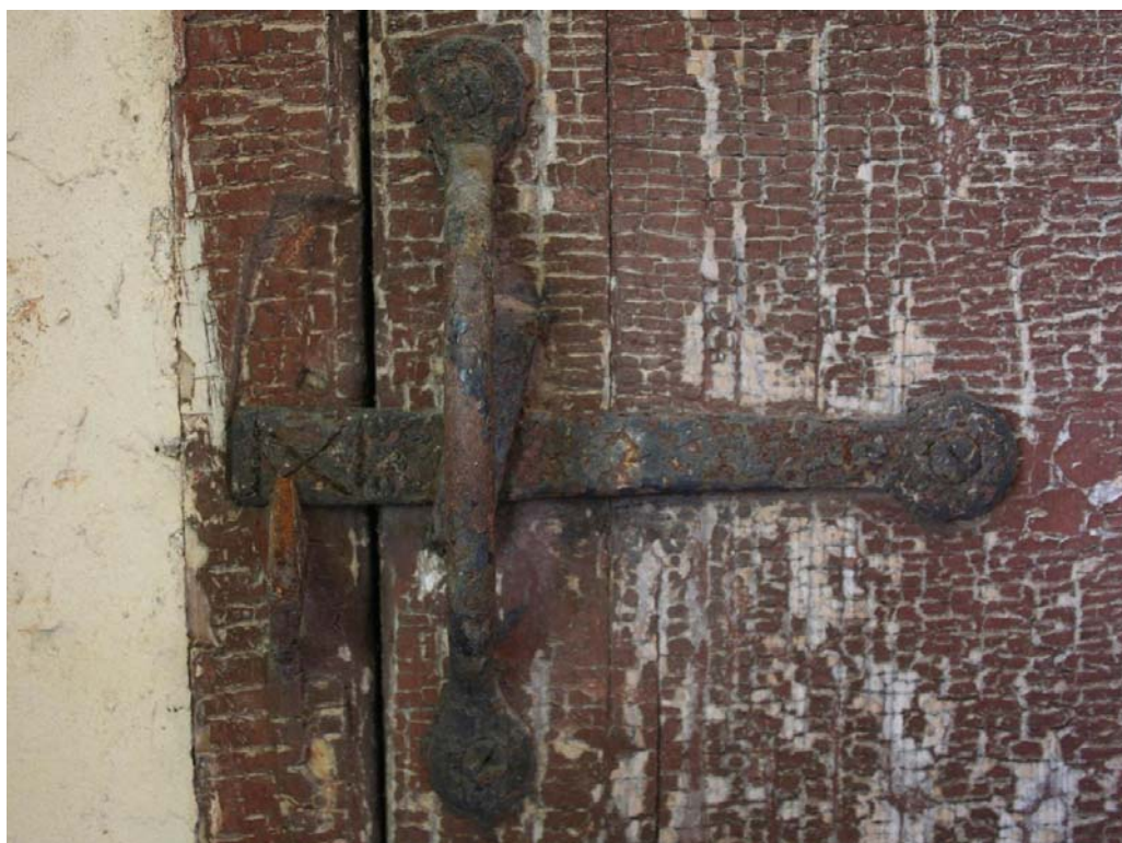
Plate 12: Ground floor interior, detail (Latch on door to storage space under stairs)
