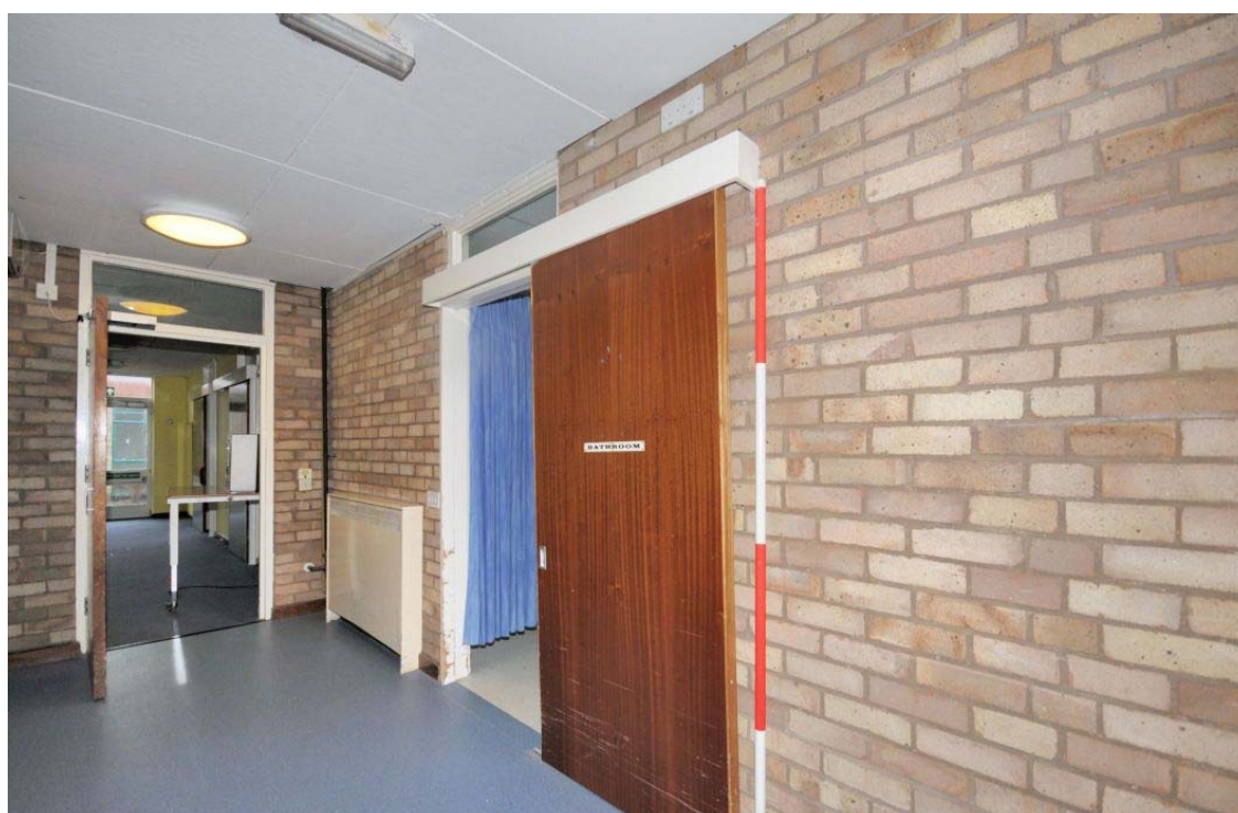
Figure 17: Cheviot residential unit, bathroom sliding entrance door
