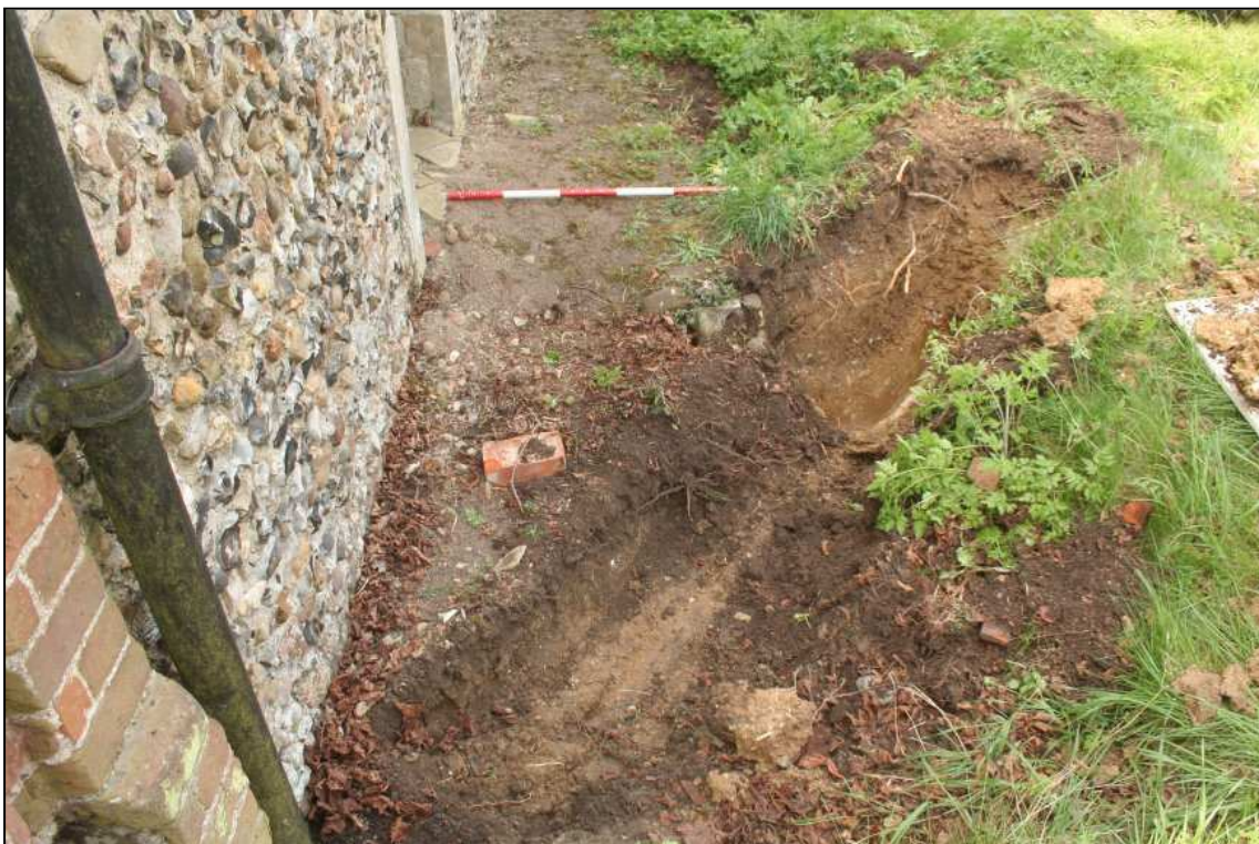
Image 6: Trench for soakaway near north-east corner of chancel, looking west (scale 1m)
