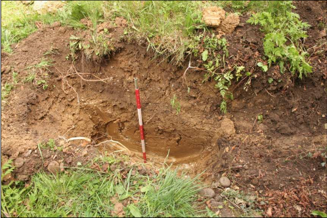
Image 7: Trench for soakaway near north-east corner of chancel, showing SW-facing section (scale 1m)
