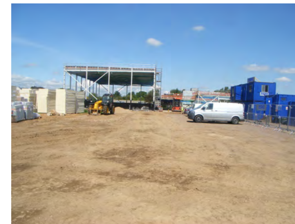
View of sports hall, site cabins (far right) and storage area (far left). Facing NW
