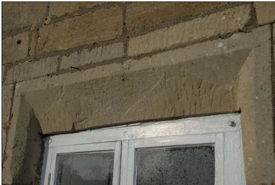
Figure 18: Detail of ground floor window in south wall of the main range
