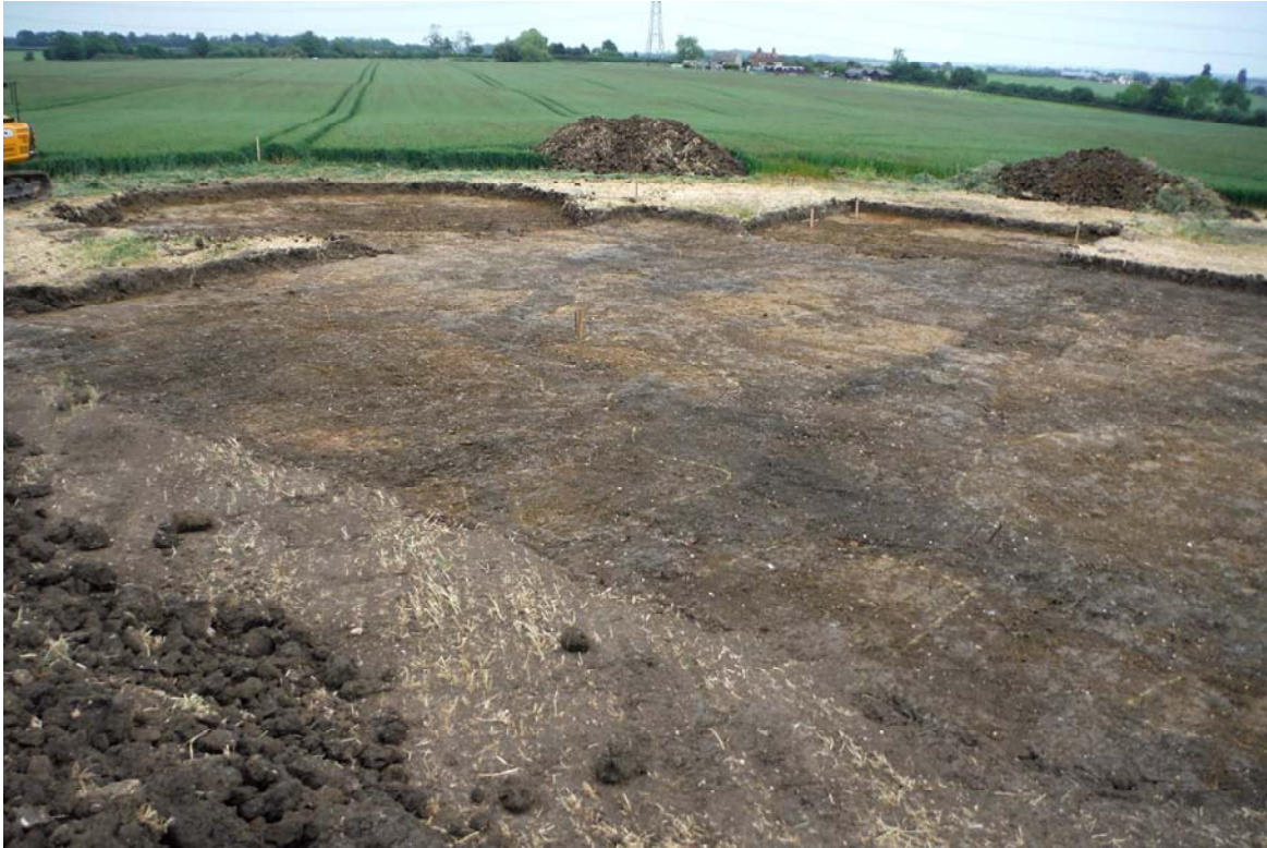
Image 1: General view of northern part of crane pad, with turbine base to top left of image and rectangular sub-station footing to right of image.
