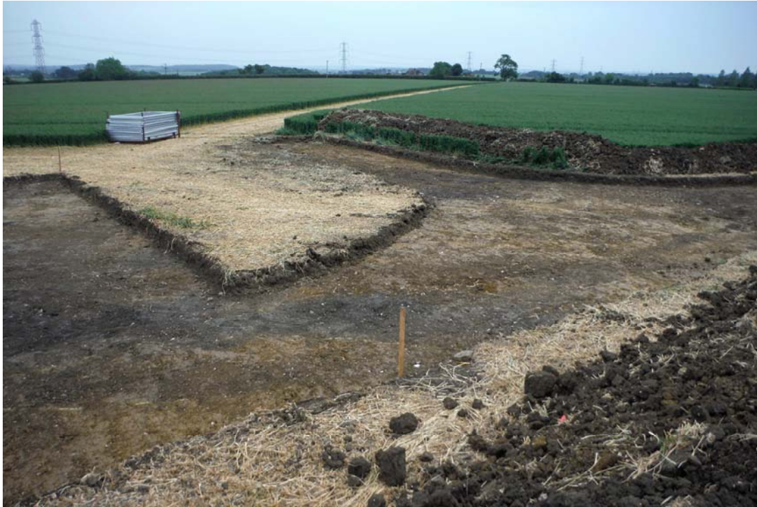
Image 3: General view of northern extent of the access road, which extends down a gentle slope to Dovecote Farm, situated off-image to the right. The crane pad is to the left of the image.
