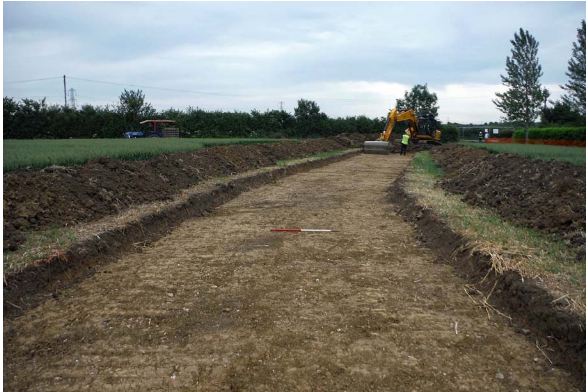
Image 7: General view along eastern part of the access road, looking towards Turvey Road. (Scale 1m in 50cm divisions)
