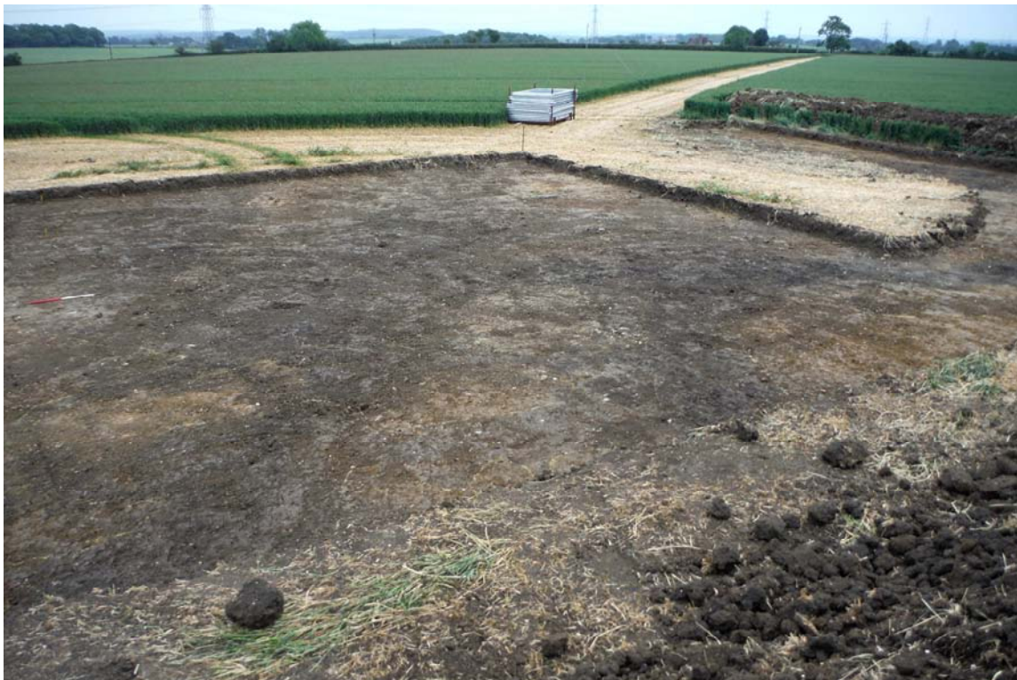
Image 2: General view of southern part of crane pad, with northern extent of access road to lower right of image.
