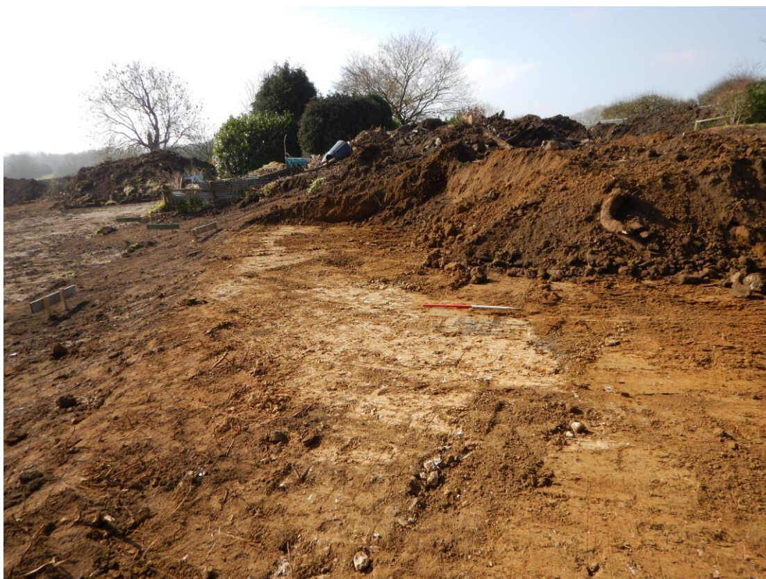
Image 3: View across partly stripped terrace with Plot 1 to the right of the image and Plot 2 on the lower ground to the left. Scale 1m in 50cm divisions.
