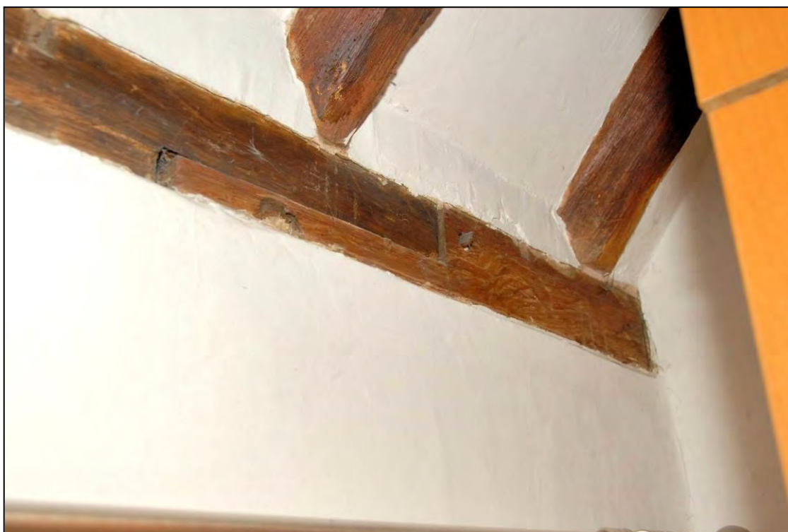
Image 16: Bedroom 1, scarf joint in wall plate
