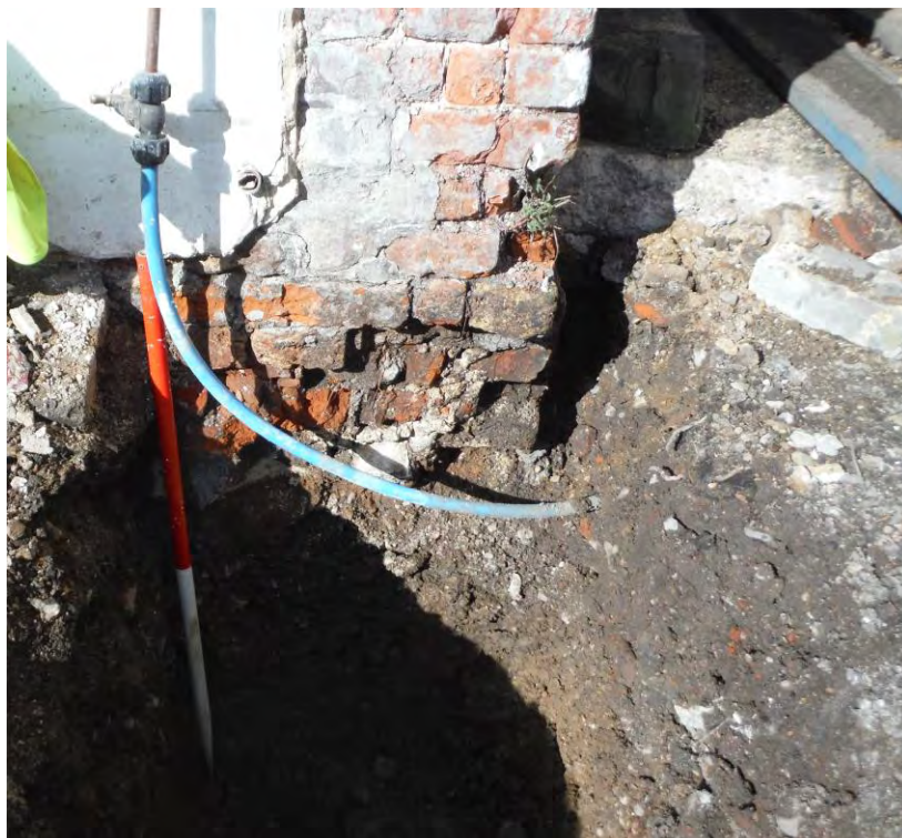
Image 31: North-west corner of cottage revealing shallower footings, which are four courses deep. Scale 1m in 50cm divisions.
