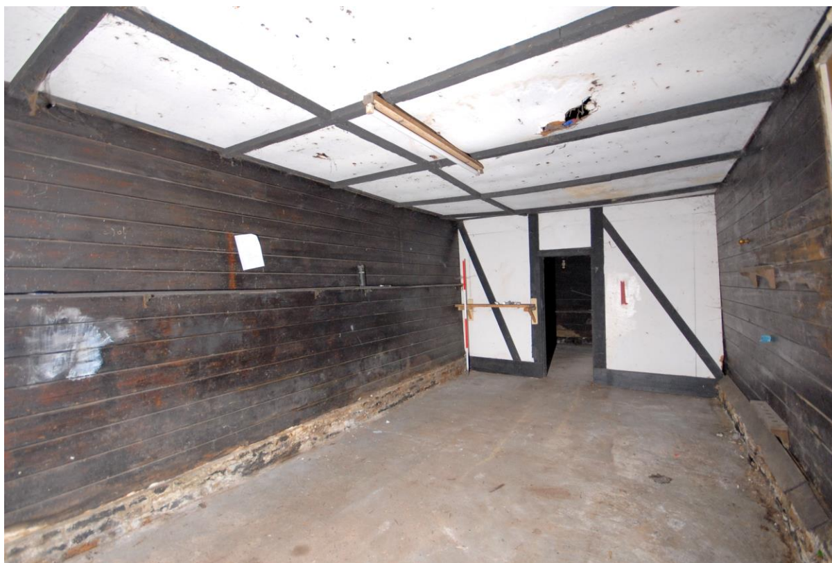
Figure 11: Southern room interior, looking NE: inserted concrete floor, ceiling and partition wall
