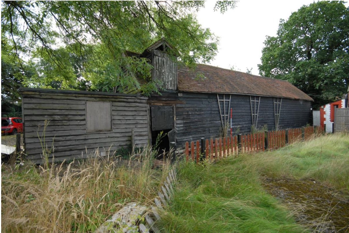
Figure 8: Former stable block NE side with flat-roofed NE extension, stable door and roof bay access
