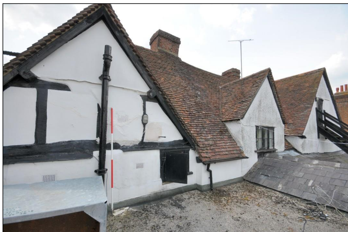
Image 4: North-east elevation of No. 69 at first floor level Seen from flat roof of modern extension at rear of property
