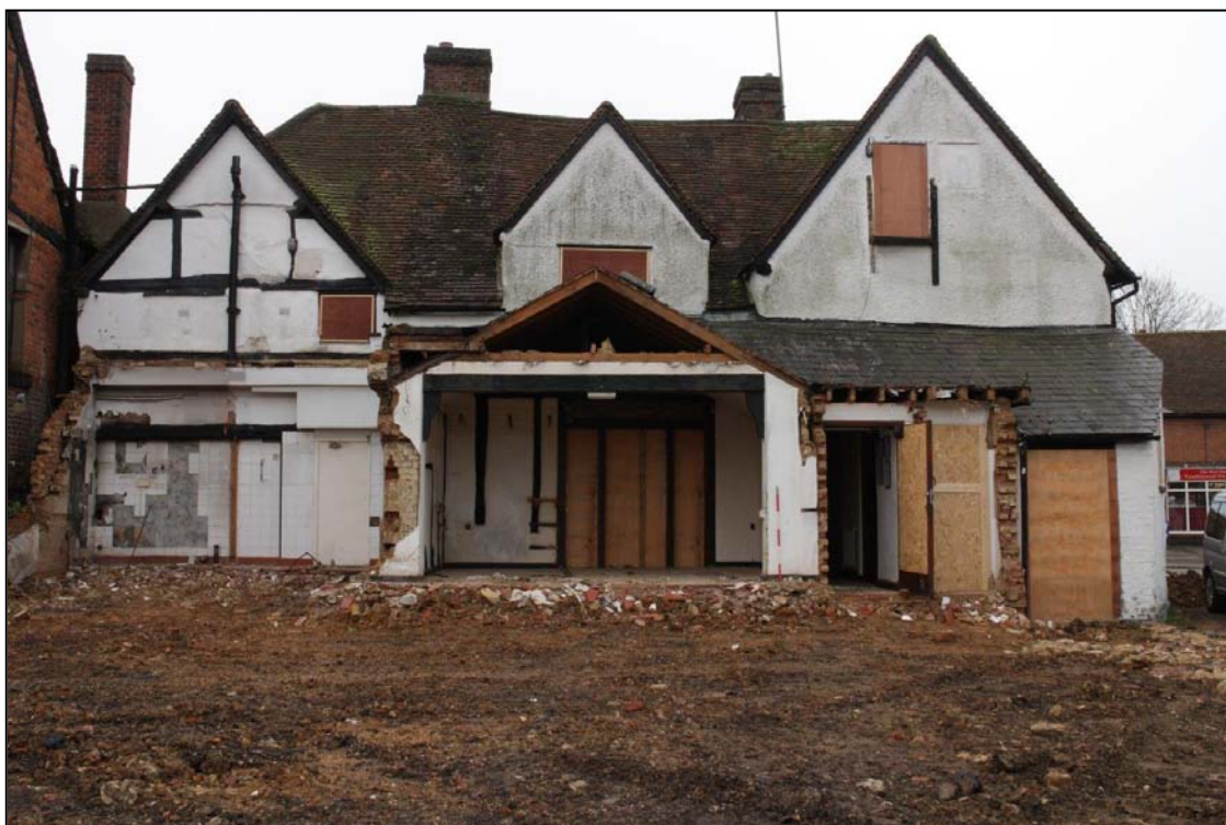
Image 35: No. 69, rear elevation after demolition of modern extension Looking south-west, showing rear elevation with north-west cross wing at right
