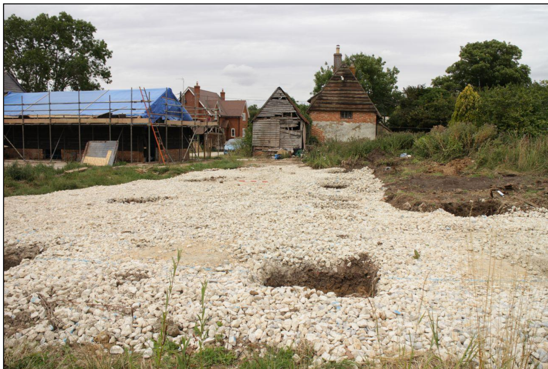
Image 3: Area 2, Wood End Farm, view of construction area Looking north-east, showing foundation pits for new agricultural building
