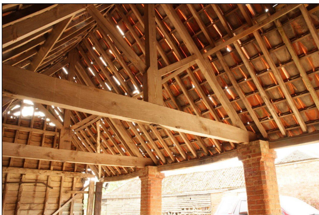
Image 16: Shelter shed, south side of roof
