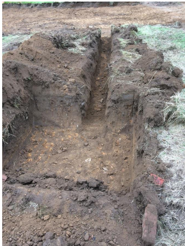
Image 2: View of soak-away pit, looking northwards to narrower drainage run and house footprint beyond.
