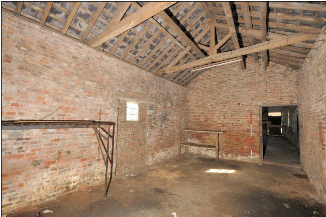
Image 33: South range: interior of compartment C7, looking south-west Showing blocked opening in south wall at left and door to compartment C8 at right (scale 2m)
