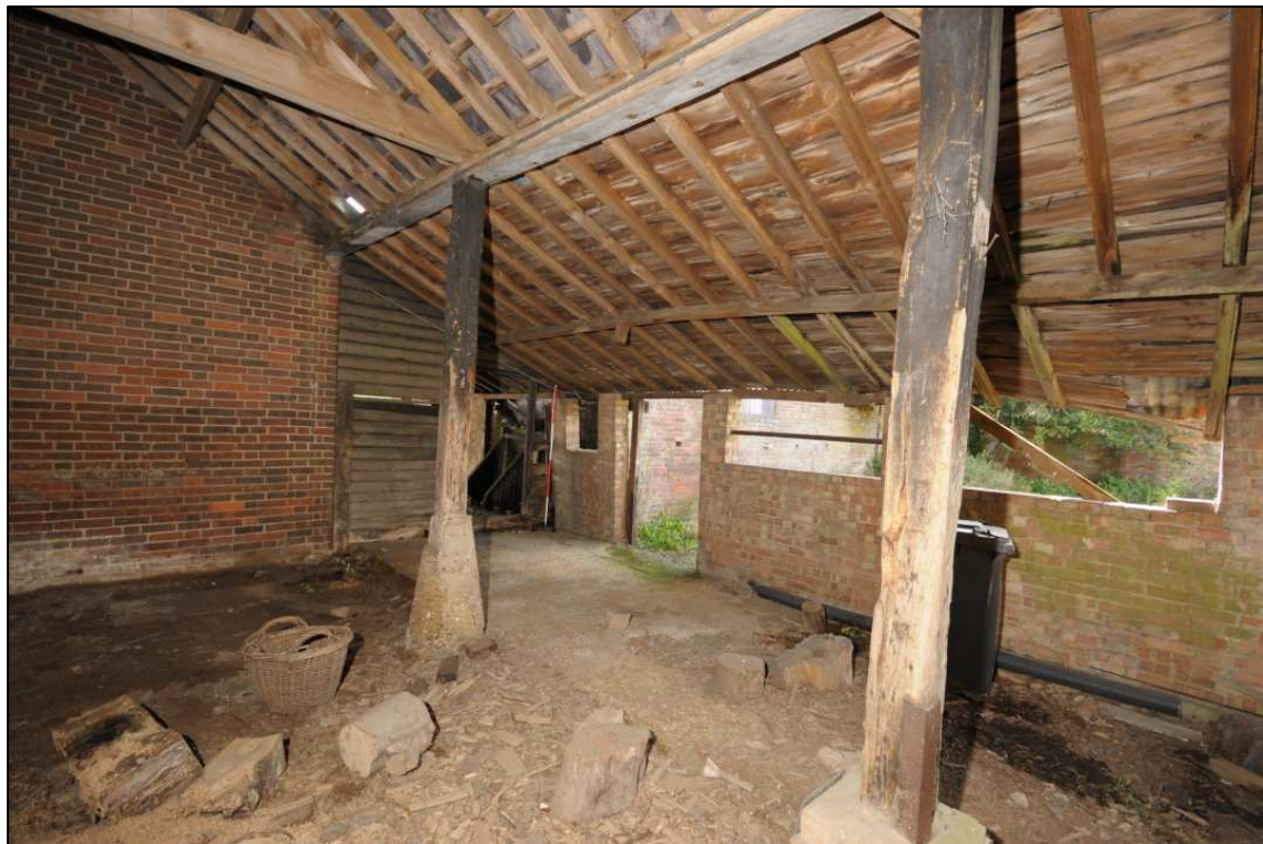
Image 18: North range: compartment C4, looking south-east View from compartment C3 showing interior of compartment C4
