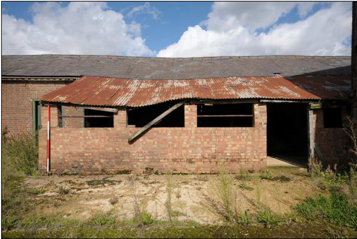
Image 17: North range: compartment C4, looking north Showing front wall with Fletton brick and corrugated iron roof (scale 2m)
