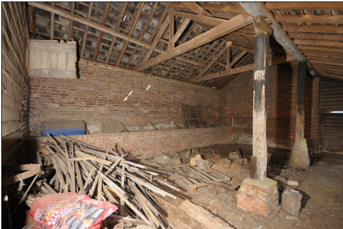
Image 14: North range: compartment C3, looking north-east Showing front supported by timber posts (scale 2m)
