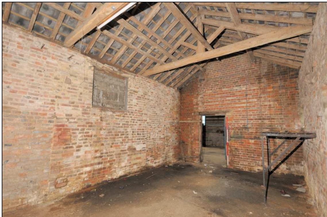
Image 34: South range: interior of compartment C7, looking north-east Showing large blocked opening in north wall at left and door to compartment C6 in end wall (scale 2m)
