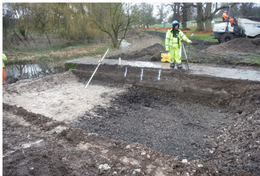
Natural geology shown to the right of picture, make up layers to the left and a large concrete drain to the rear (looking SE)
