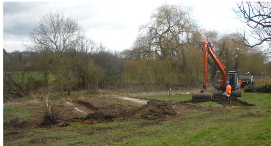
Wetland area, with tree removed and modern concrete drains exposed; service trench being opened (looking SE)
