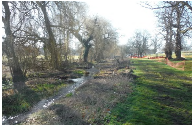
River channel and terrace cleared of vegetation and weir removed (looking SE)
