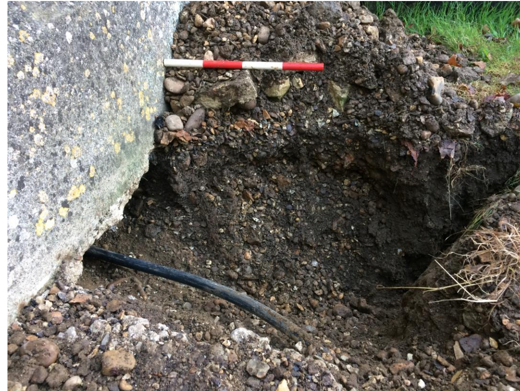
Plate 6: Trench 1 – water pipe connection point, old service pipe and gravel-filled French drain (scale 40cm)
