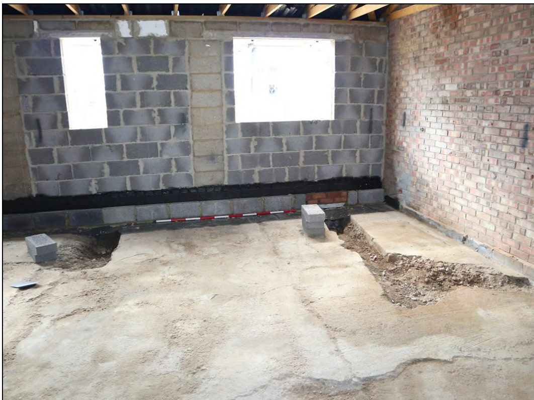
Image 4: Service trenches in east side of the workshop (Looking south-east, scale 2m)
