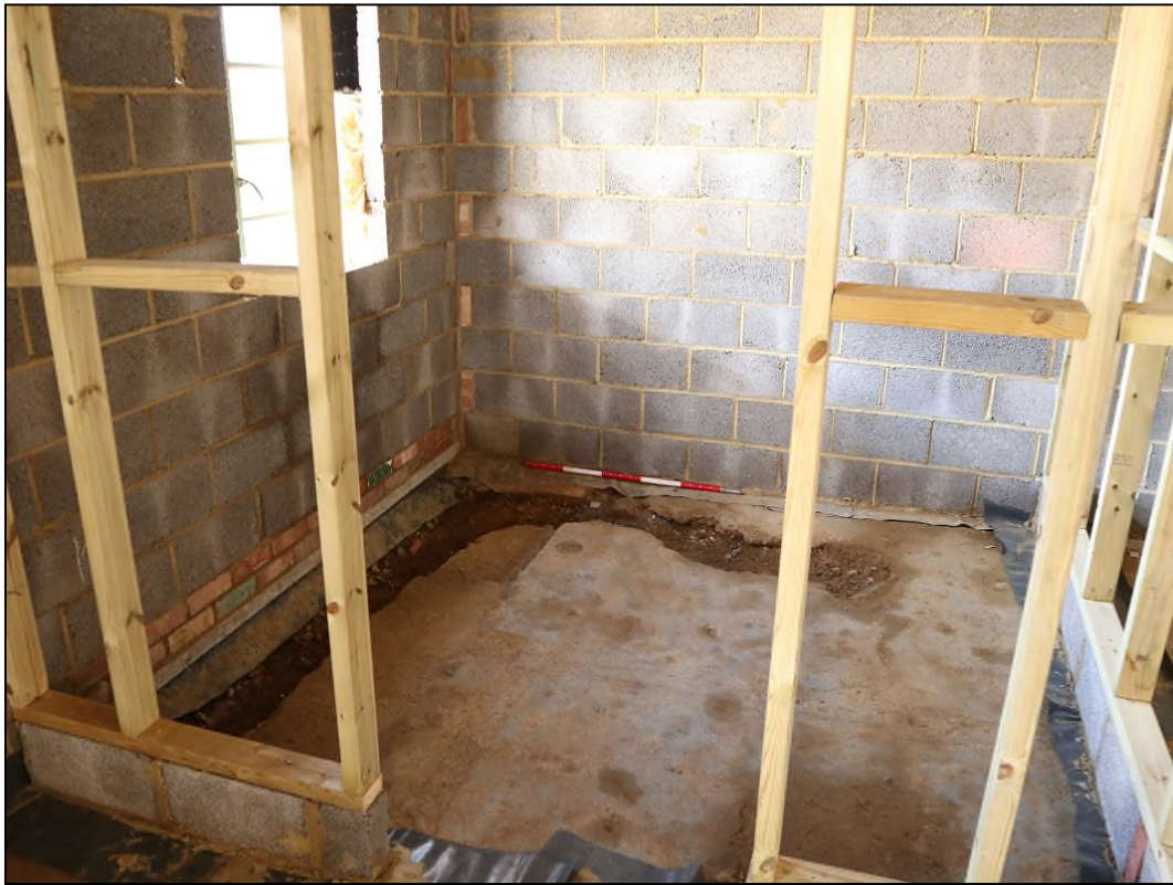
Image 3: Service trench in north-west corner of the workshop (Looking north, scale 1m)
