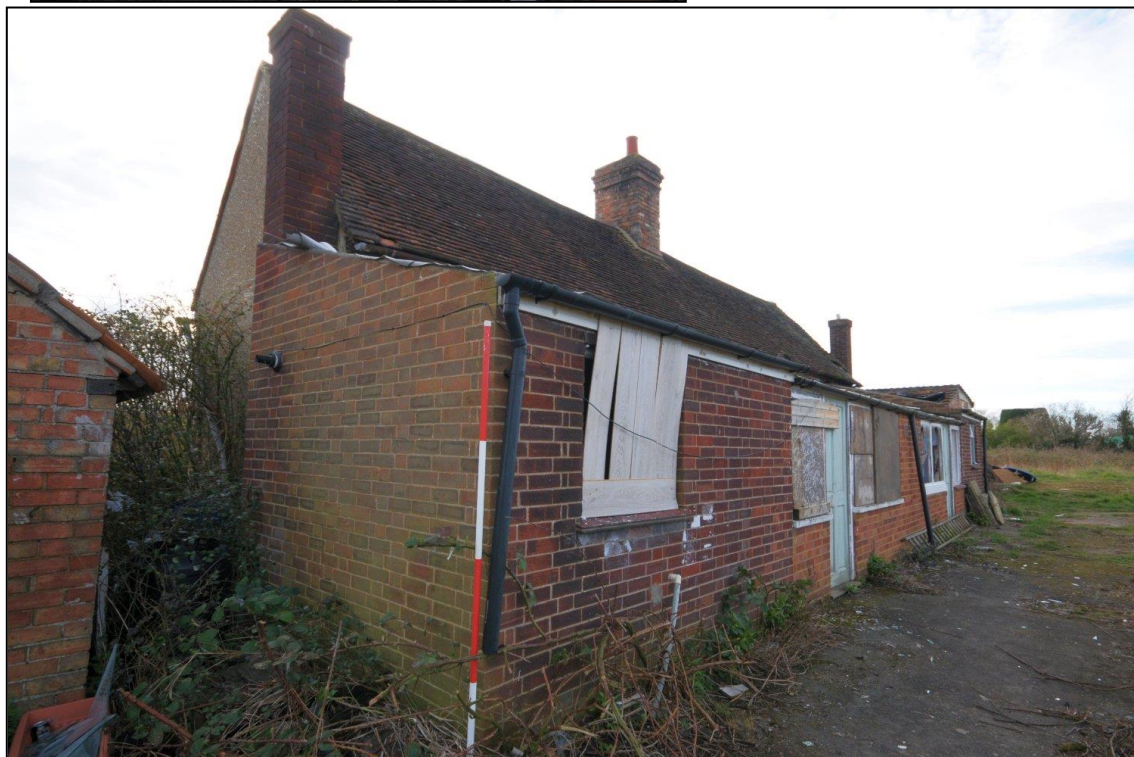
Image 6: Rear elevation, viewed from north-west Lean-to extension of No. 43 in foreground (Scale 2m)
