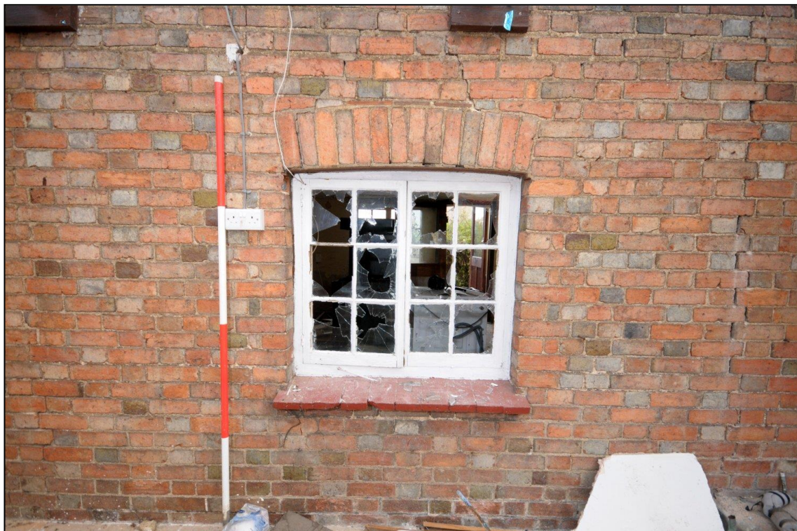
Image 18: No. 41, conservatory, detail of window Rear window in primary range (Scale 2m)
