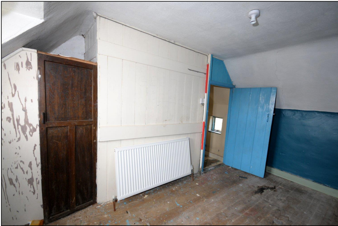
Image 49: No. 43, bedroom 2, looking south-west Boarded partition with later wardrobe at nearest end (Scale 2m)
