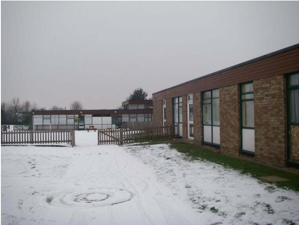
Figure 4: Brick residential block (foreground) and steel framed teaching block (background). Original metal frames and PVC replacements are in evidence in teaching block.
