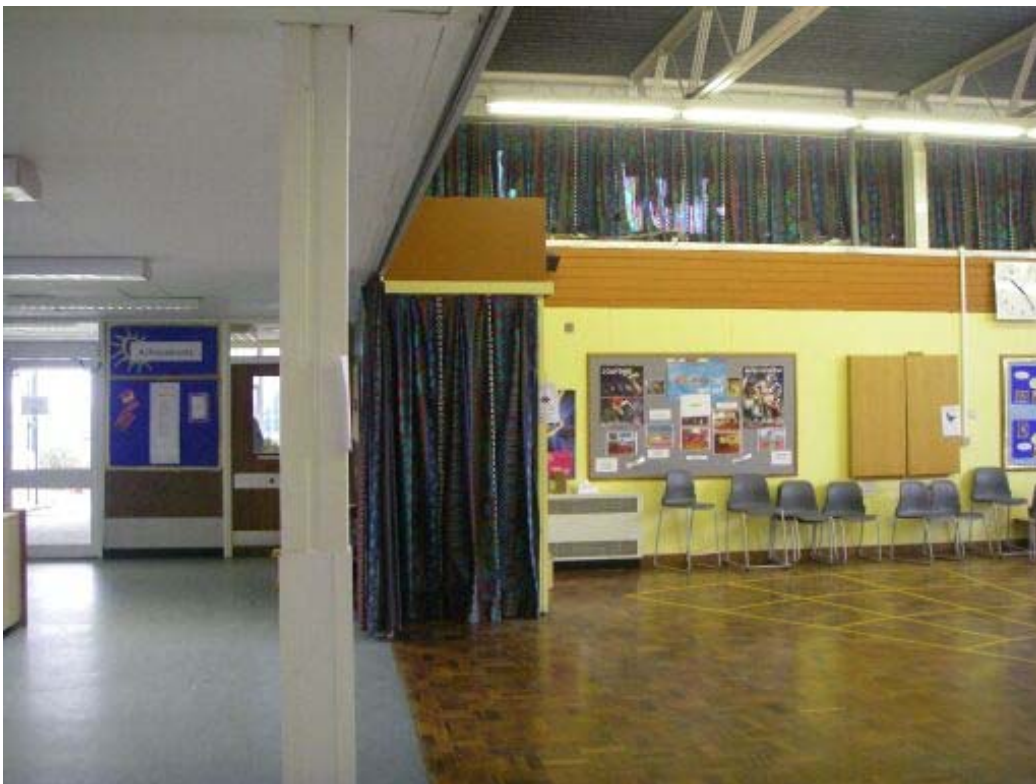
Figure 5: Assembly hall and central access spine. Lattice beams are visible in ceiling of assembly hall.
