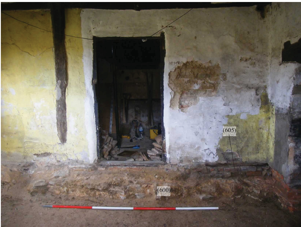
Photo 10: Foundations of the north-east wall in the 'kitchen' of the lobby-entry dwelling
