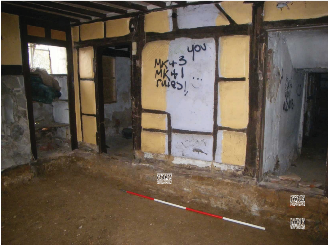
Photo 11: Foundations of the south-east end of the lobby-entry dwelling visible from inside the end-stack dwelling (Photo digitally altered to remove obscene Graffiti)
