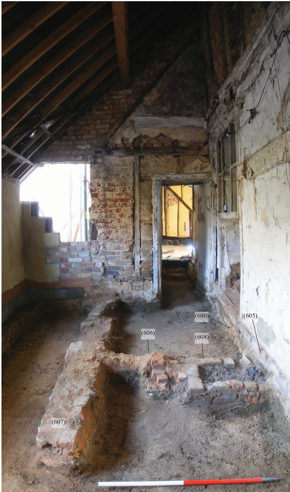
Photo 15: Foundations and ‘ash chute’ collection box within the ‘pantry’ extension (Several phases are visible in the walls behind.)
