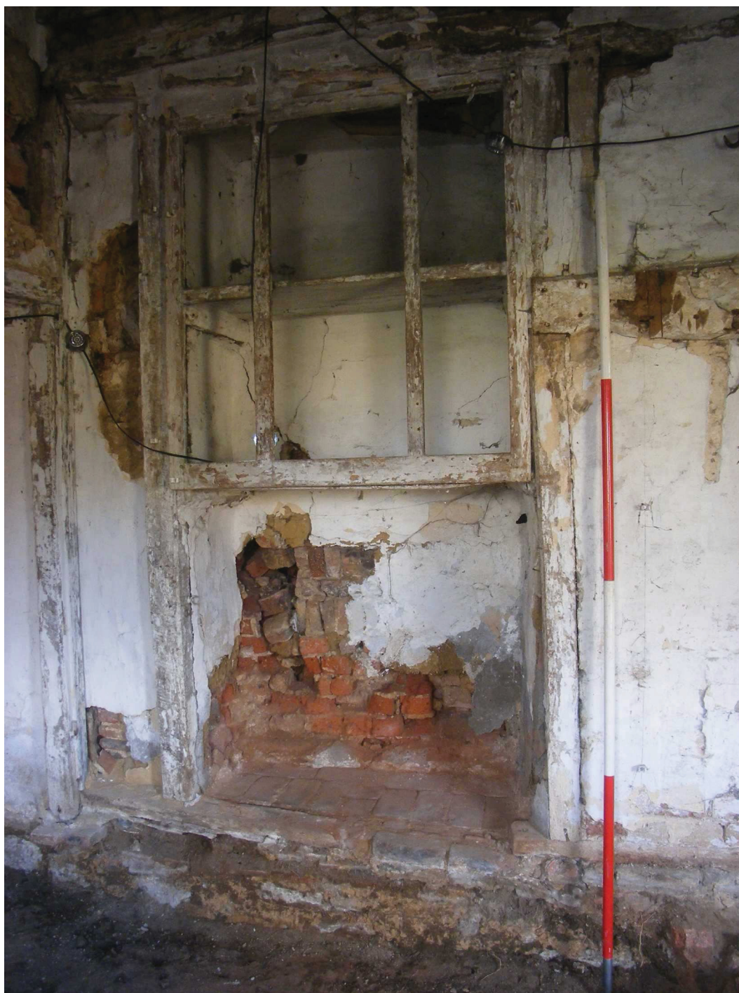
Photo 18: Former opposing door of lobby-entry dwelling that was later blocked by the addition of the fireplace (The recess was converted into a cupboard)
