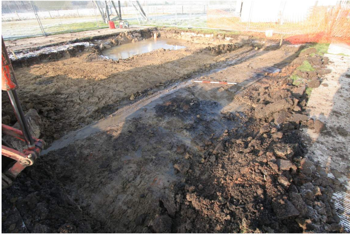
Image C: View of trench looking north-west (Shows area of burnt clay and charcoal just in front of 1m scale, linear cut for modern ducting and water-filled depression where concrete road has been removed)
