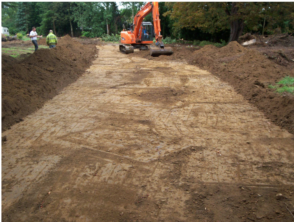
Image 1: Stripping of the driveway down to formation level, revealing the interface between ploughsoil and underlying subsoil.
