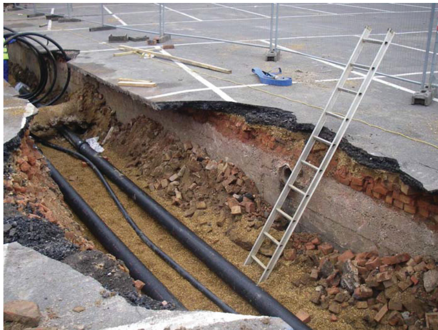
Image 2: Trench in car park showing King's Ditch culvert A concrete culvert enclosing the King's Ditch is visible in the east side of the trench
