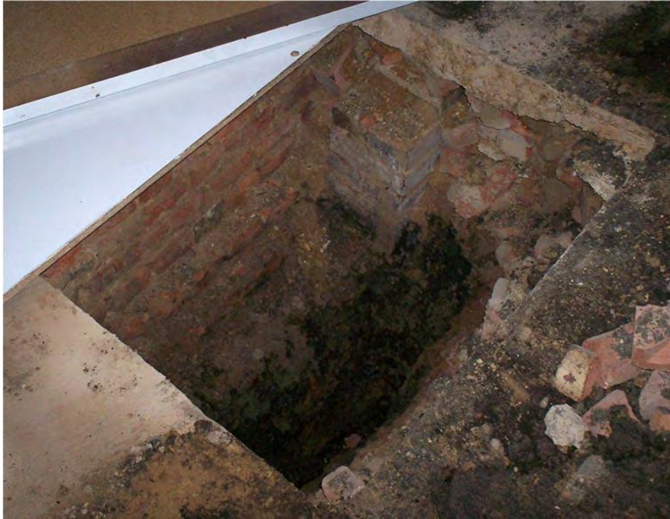
Image 1: Stepped footings of brick partition wall. The black deposit below the rubble is coal dust, suggesting that a coal cellar occupied the area towards the street frontage.
