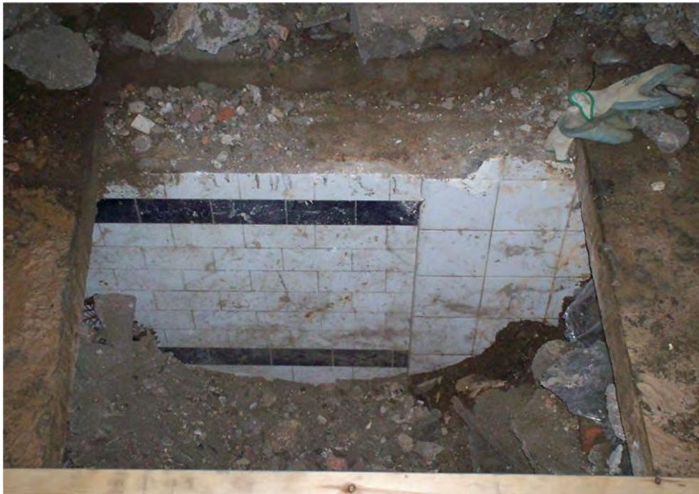
Image 2: Evidence for a second cellar revealed toward rear of building. The change in tiles may suggest a subdivision of this area.
