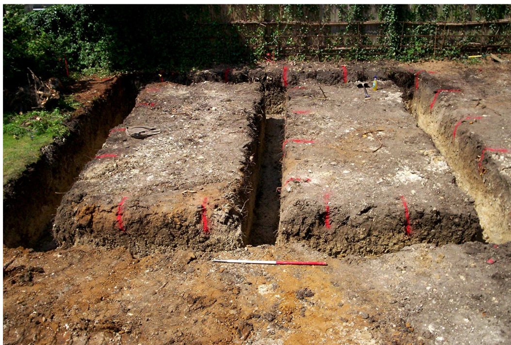
Image 1: General view of excavated garage footings, looking west. Scale 1m in 50cm divisions.
